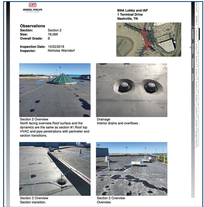
Figure 5 – FCS standard observation overview page at the beginning of a detailed roof report. Gives the client a general overview of conditions observed that don't necessarily need correcting.
