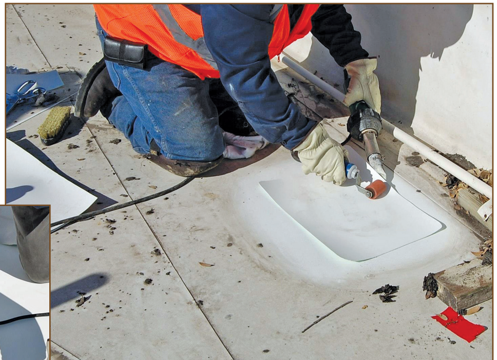
Figure 5 – Repair of aged TPO membrane with a new patch welded to the aged cap. Image courtesy of WSRCA.
