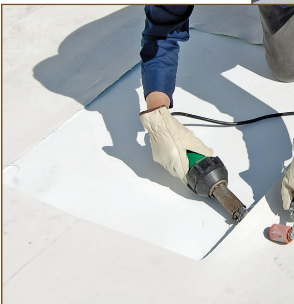
Figure 6 – Repair of aged TPO membrane with a new patch welded to the aged core. Image courtesy of WSRCA.
