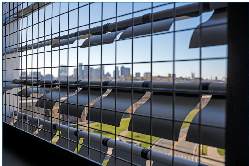
Figure 4 – Logan International Airport’s Walkway and West Garage features a wind-driven kinetic façade system with 48,000 aluminum flapper panels to screen the parking structure. Designed by architectural firm Arrowstreet Inc. in collaboration with façade manufacturer EXTECH, the garage’s dynamic wall enhances the view for the traveling public.
