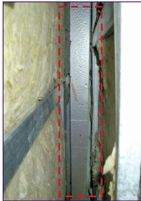
Figure 10 – Looking up inside a balloon-framed parapet with condensation at the top of parapet from interior conditions. (Image adapted from the U.S. Environmental Protection Agency – Moisture Control Guidance for Building Design, Construction and Maintenance.)
