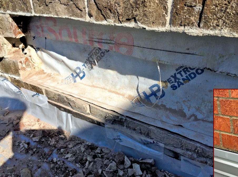
Figure 3 – Picture of failed through-wall membrane without through-wall metal.
