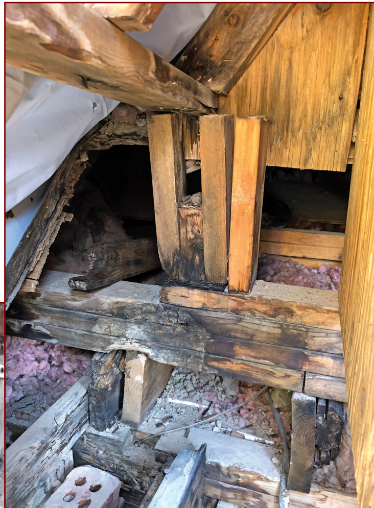
Figure 6 – Picture of framing damage due to improper flashing.
