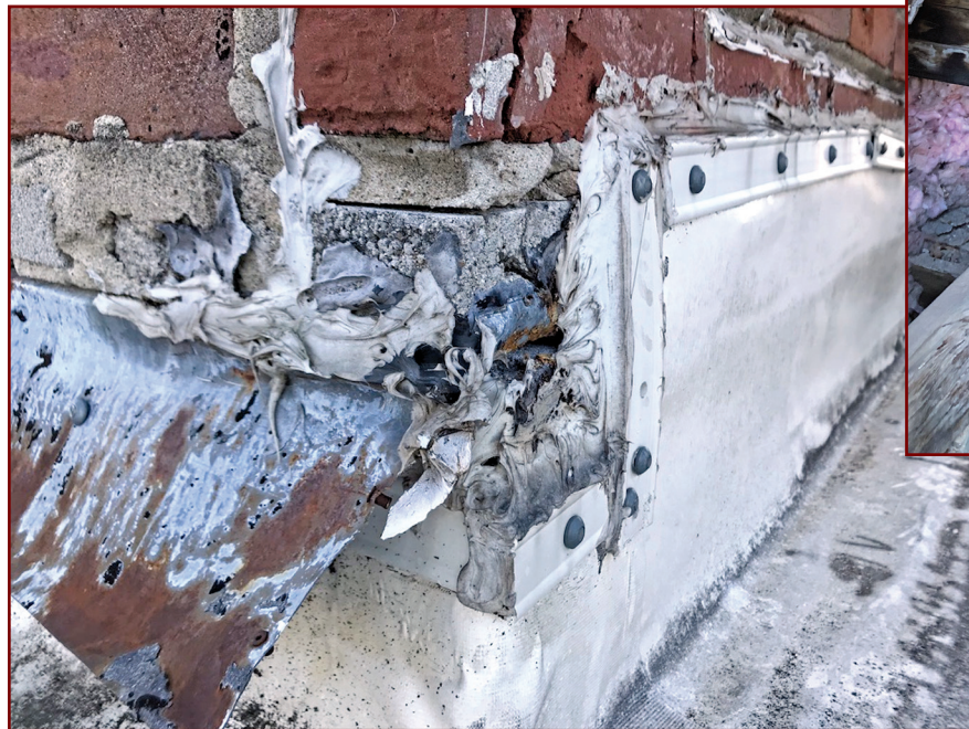
Figure 5 – Improper wall termination.
