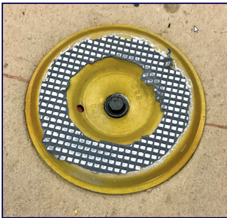
Figure 8 – The top of an induction weld fastener plate showing membrane delamination (cap-to-core separation).
