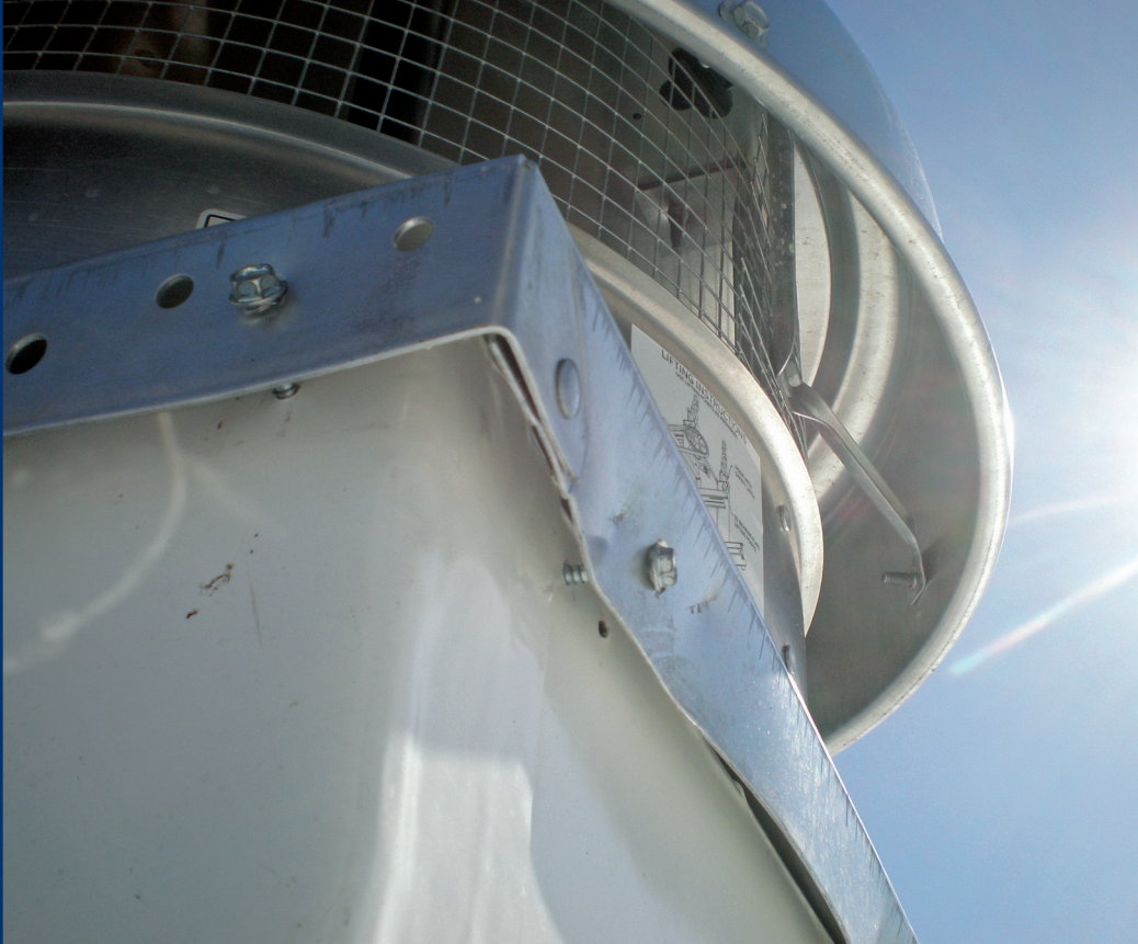
Figure 10 – Gap between downturned flange of exhaust fan and base flashing.
