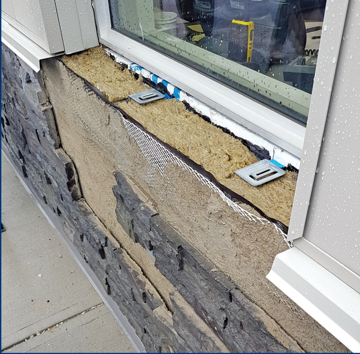
Figure 14. Exterior insulated steel-stud wall assembly clad with adhered manufactured thin-stone masonry veneer.
