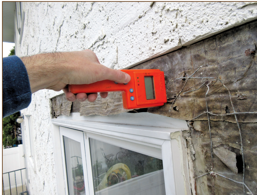
Figure 4 – Photo of a cementitious stucco cladding system over a concealed barrier. Note that drainage is provided behind the cladding via the use of a weather-resistive barrier, lapped over the window head flashing to facilitate drainage.
