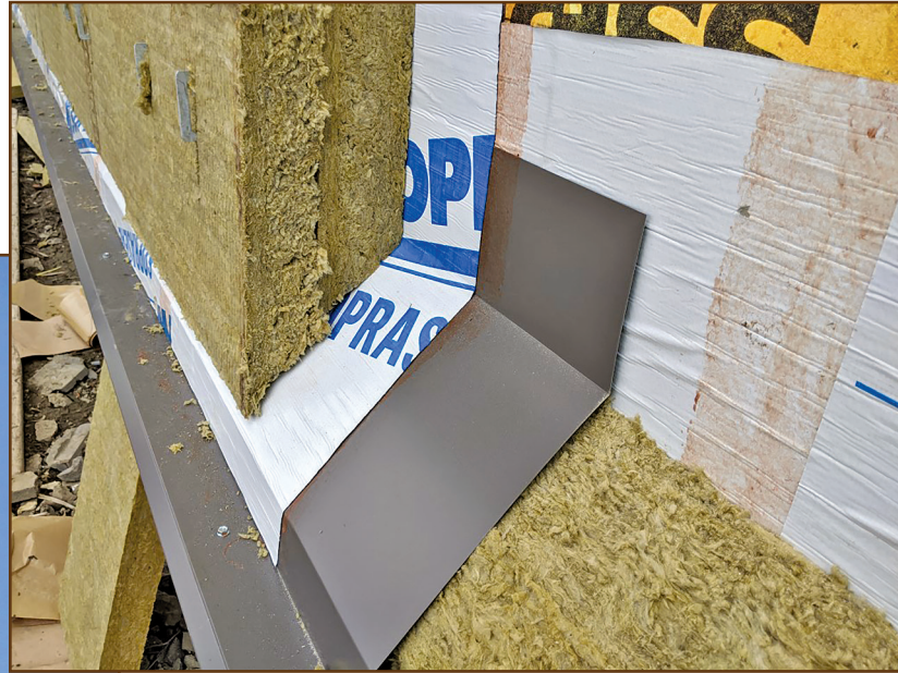
Figure 6 – Photo of a cross section of a drained and vented masonry-veneer wall assembly under construction.
