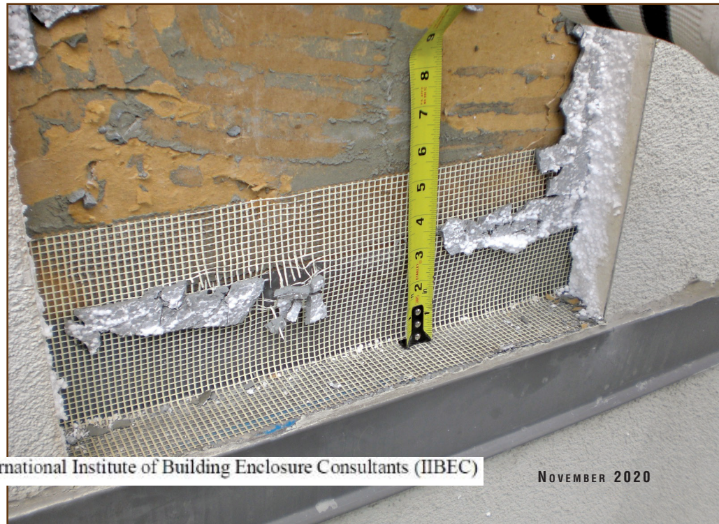
Figure 2 – Photo of a face-sealed exterior insulated finish system (EIFS) cladding. Note that the base of wall at the flashing is sealed and that there is no allowance for drainage behind the cladding system.
