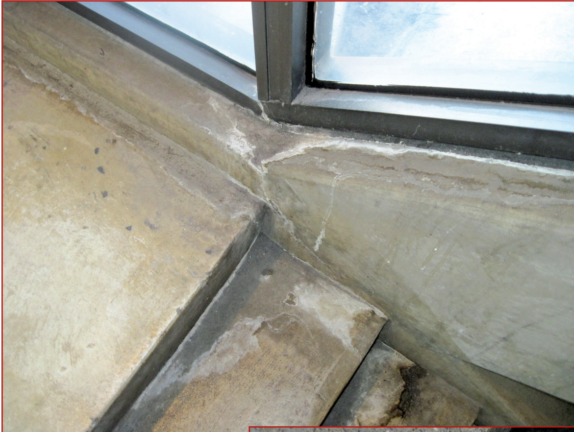
Figure 4 – Through-wall cracking and failed sealant resulted in leakage at this concrete stairwell.
