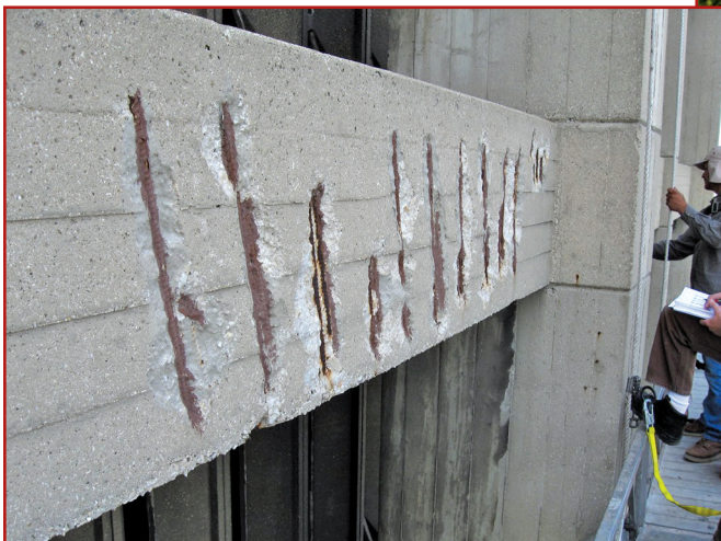
Figure 1 – Spalled concrete and exposed reinforcement bars observed during a façade investigation. Many bars had less than ½ in. of concrete cover.
