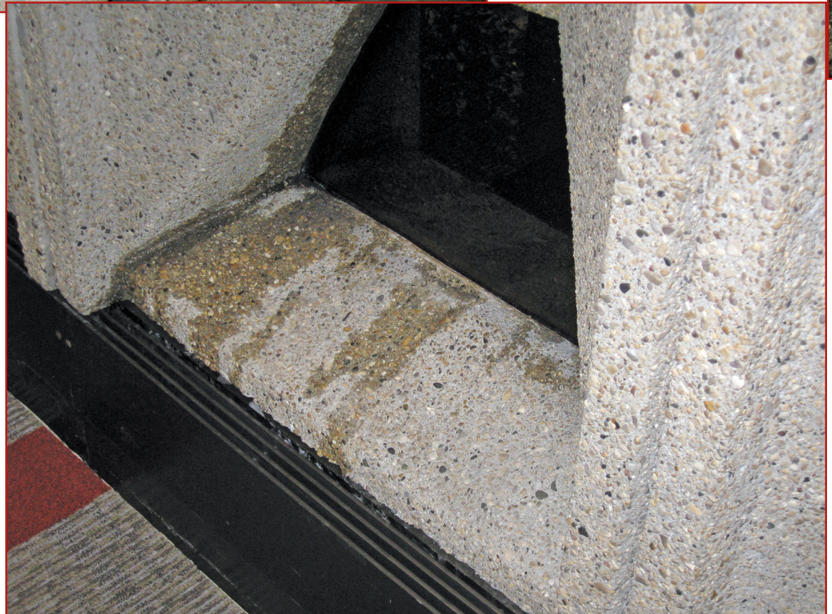
Figure 5 – Interior leakage at precast concrete window system.
