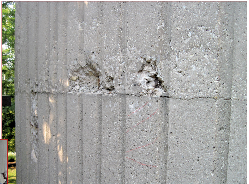
Figure 2 – Concrete spalling observed during investigation of a concrete façade.
