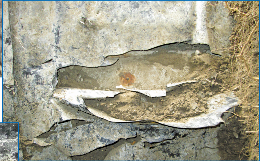
Figure 12 – Contractor(s) severely damaged the sheet membrane during the backfilling process.
