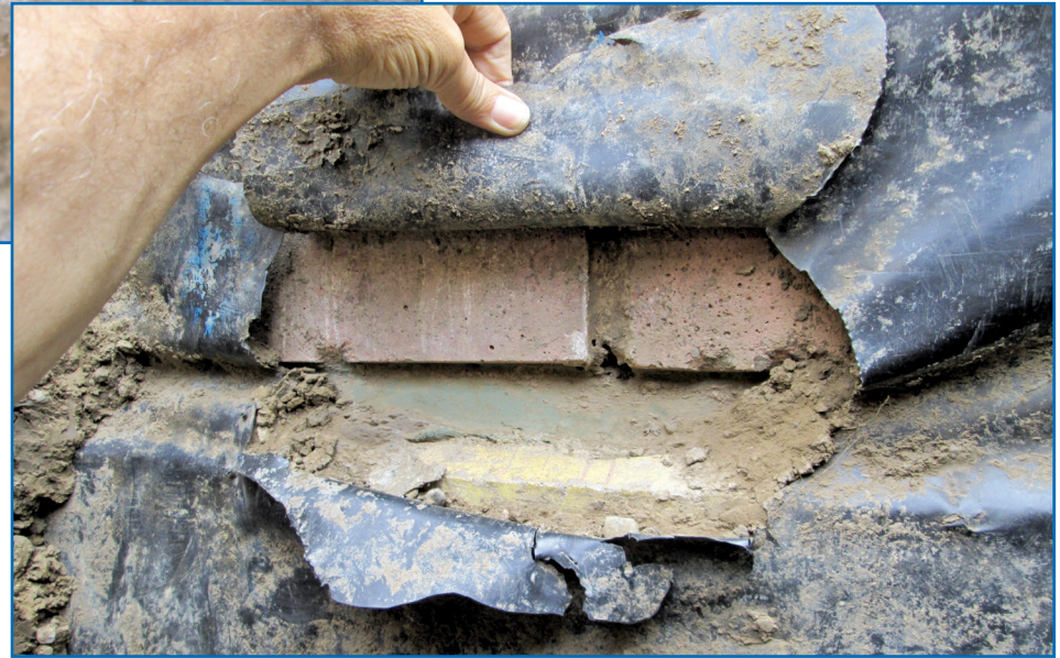
Figure 13 (very near the bottom), contractor(s) had extensively damaged the sheet waterproofing membrane during the backfill process.
