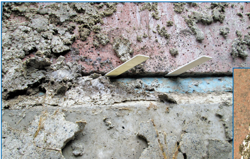
Figure 10 – The caulk joint between the two wall systems was not watertight due to failed bonding at the precast panels.
