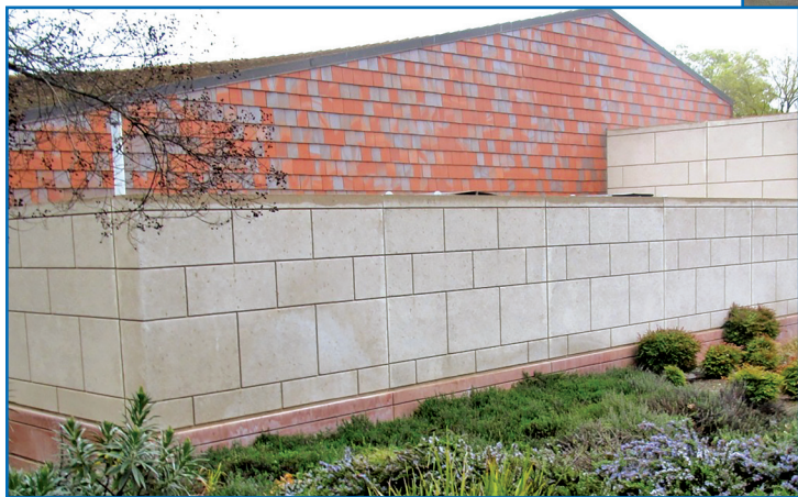
Figure 1 – Boiler room has perimeter cast-in-place concrete walls (commencing below the reddish precast panels) extending down to the concrete footings. (Whitish precast concrete panels extend up from the red panels.)
