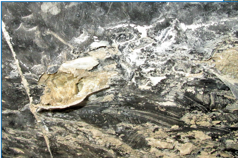
Figure 13 – (below) Near the bottom of the excavated trench, breaches in the waterproofing still remained prevalent.
