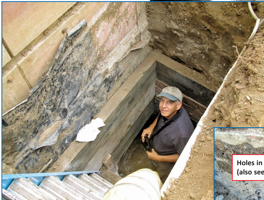
Figure 5 – Upon commencing the excavation process, a raggedy, poorly attached, and extensively torn sheet waterproofing membrane was exposed. (The missing section at the top of this photo was extracted by our crew for sampling purposes.)
