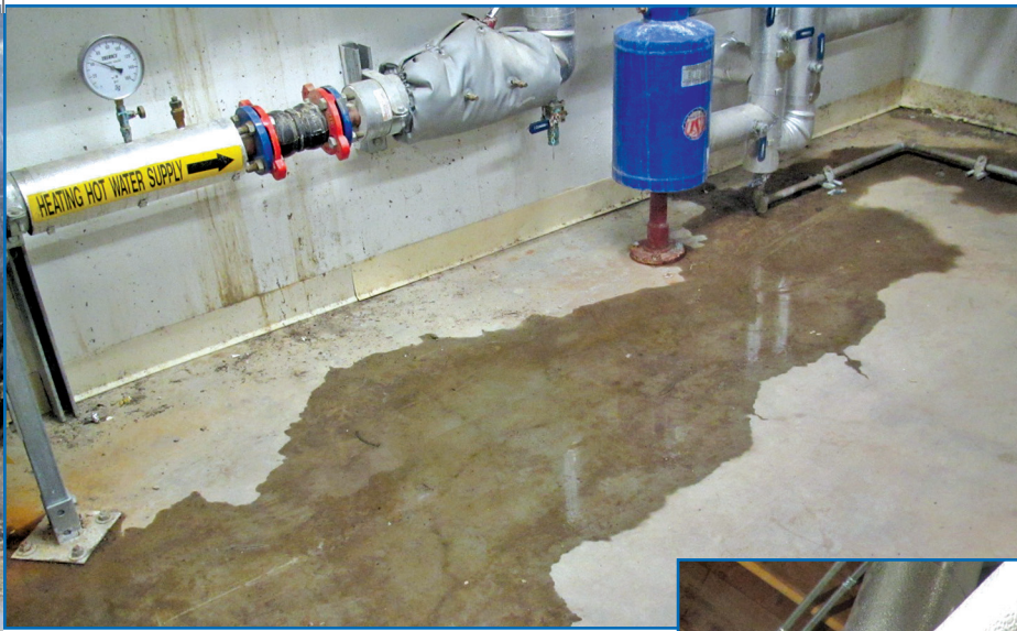
Figure 3 – Even during dry weather, groundwater infiltrated the boiler room at floor-to-wall transitions. The water stains at the lower cast-in-place wall (at left) resulted from leakage occurring at the top of the concrete wall (see Figure 4).
