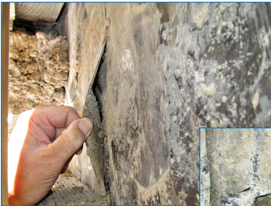
Figure 11 – Multiple breaches in the membrane due to damage during backfilling were observed at all levels of the excavation.
