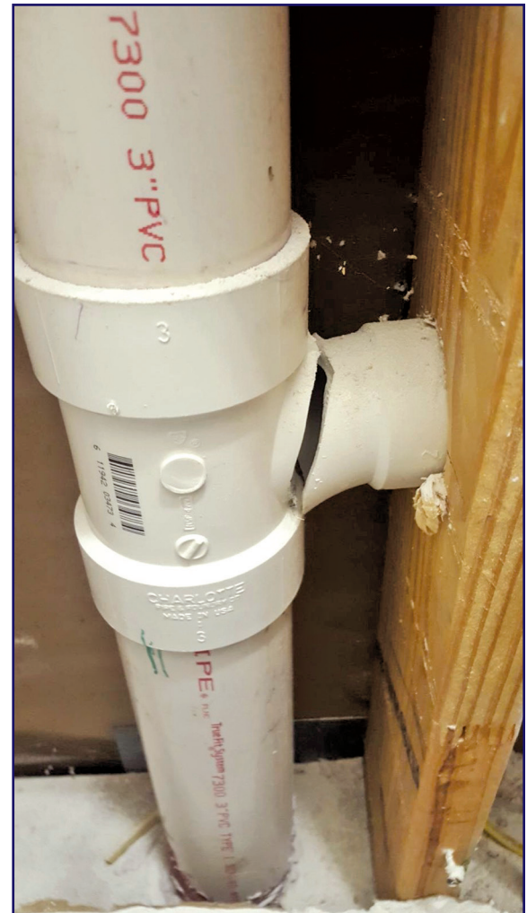
Figure 6 – This photo shows damages to PVC pipe caused by wood shrinkage.
