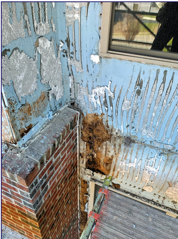
Figure 4 – This figure shows concentrated water intrusion and associated damage.
