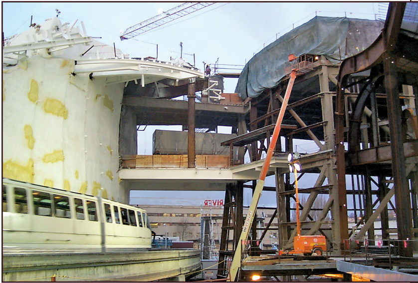
Figure 5. Photo shows acrylic coating, SPF exposed at repairs, and active monorail. Photo courtesy of MoPOP staff.
