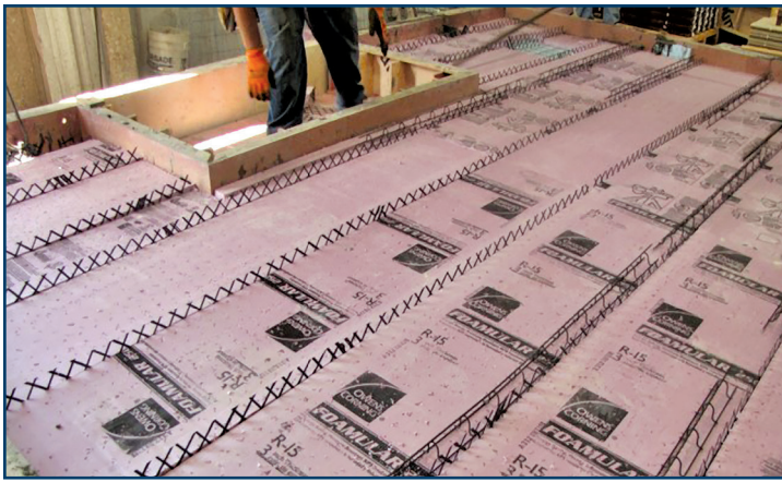
Figure 4. Roughened XPS insulation is placed in the formwork prior to concrete placement.
