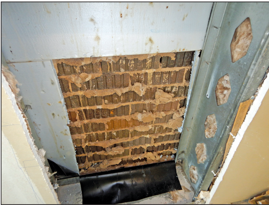
Figure 5. Forensic study image where the brick cladding was inspected from the inside of the building by removing interior finishes and sheathing. Note through-wall flashing at bottom of photo.
