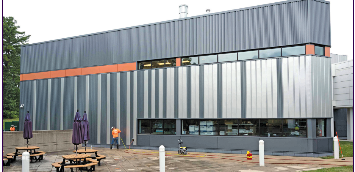
Figure 15. Another view of the completed end wall with custom colors and variation of metal building wall panels.
