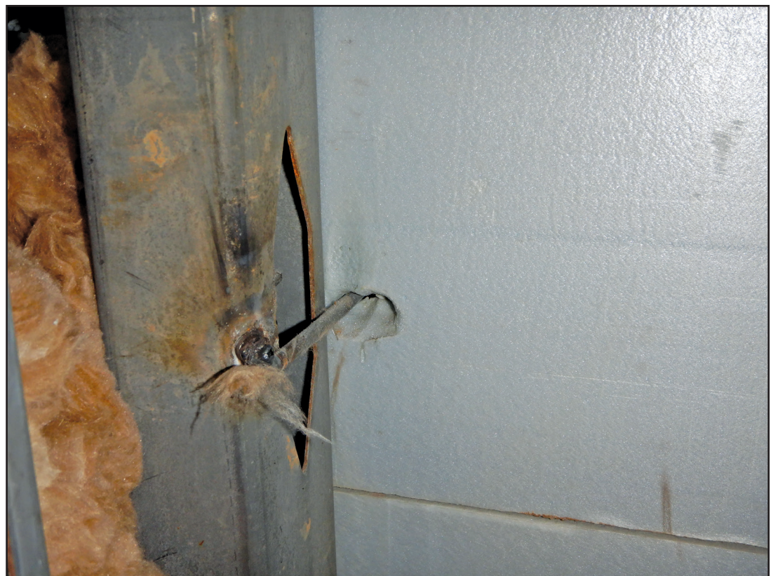
Figure 6. Forensic image of one of the methods used, fastening brick cladding anchors to the steel studs where the anchors were field-welded in place; note large hole melted in the foam sheathing.
