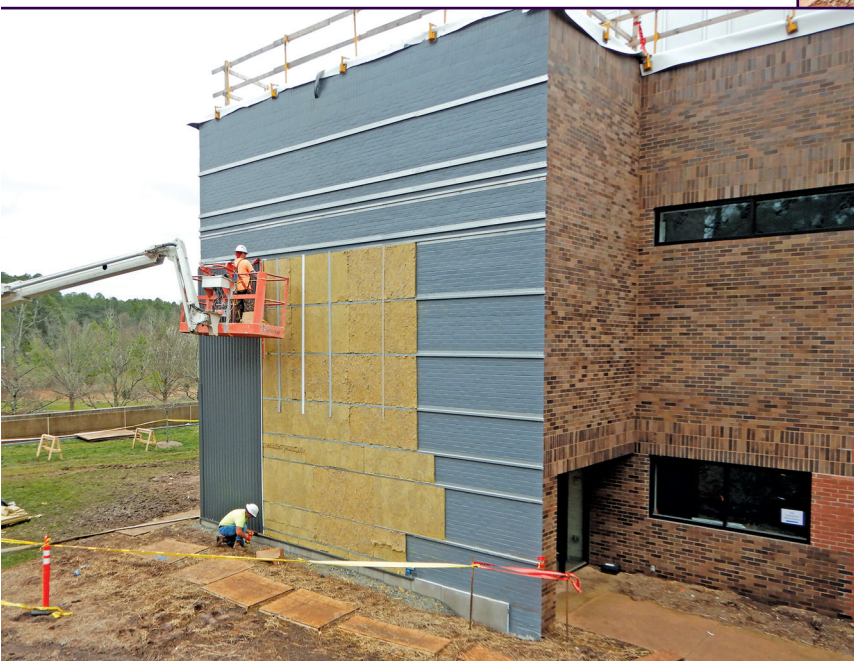
Figure 10. Ongoing work where the liquid-installed air barrier is visible, as well as horizontal Z tracks and thermal insulation prior to installation of metal wall panels.
