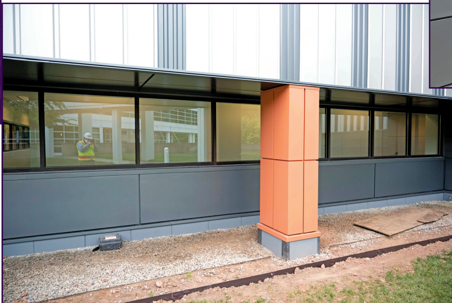
Figure 12. Finished metal cladding system depicting custom colors and variation of panel types and details.
