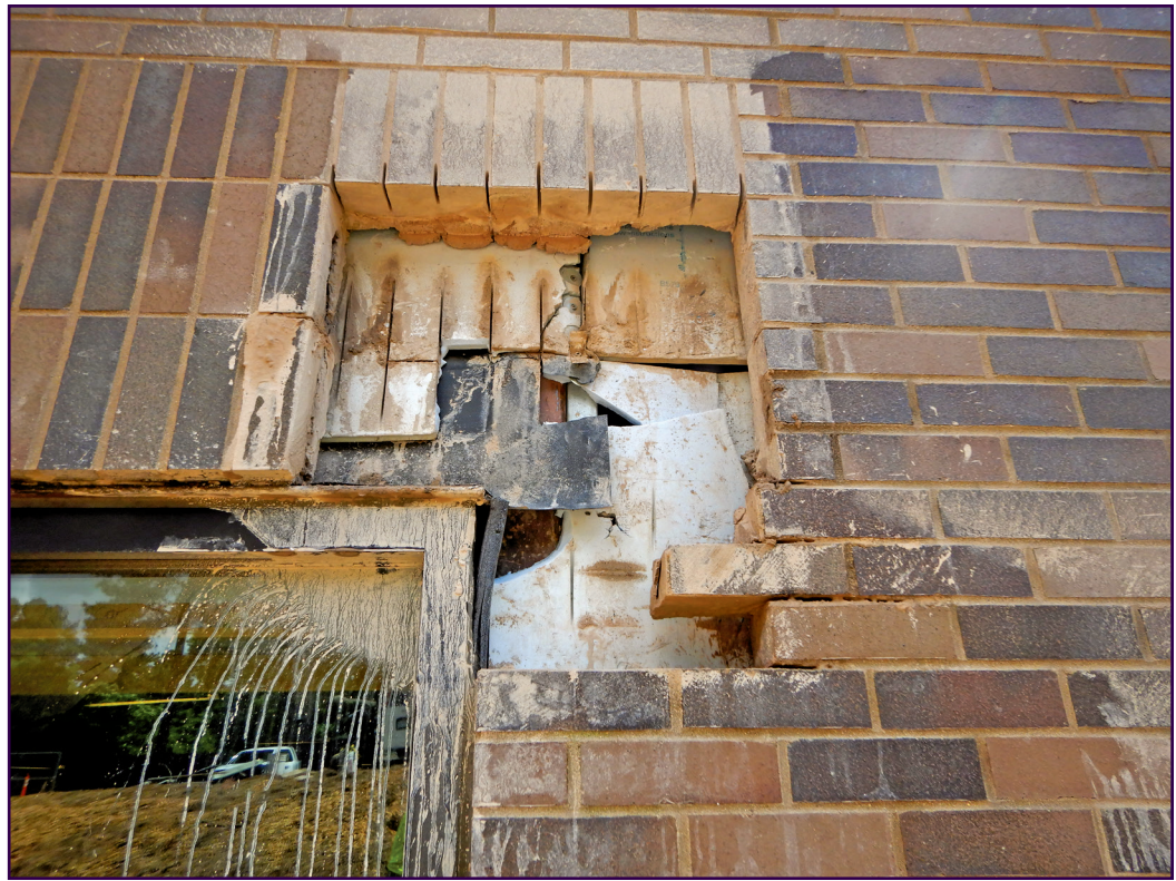
Figure 4. Inspection location at a window head corner revealing the condition of the loosely placed rigid foam board sheathing and poorly installed PVC flashing.
