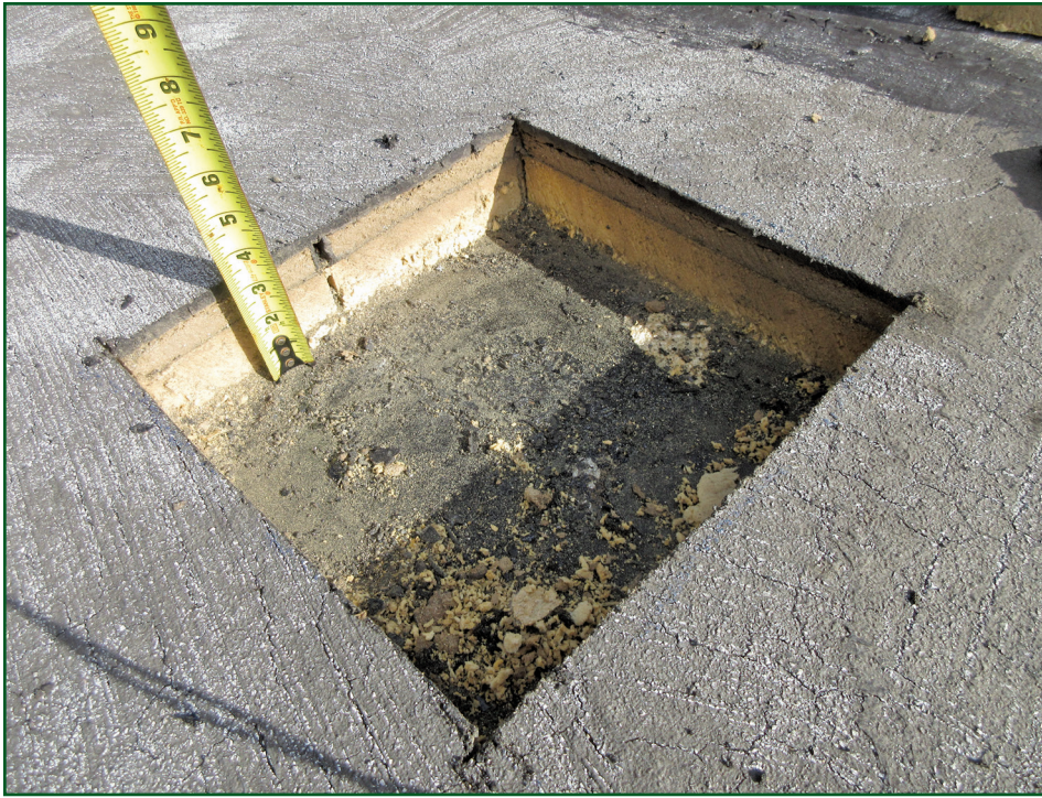
Figure 1. Core cuts or larger destructive openings into the existing roof assembly can be used to confirm components and condition of the in-service roof system as well as results of non-destructive testing. This information will help the design team and owners define necessary repair or replacement scope criteria early on in a project.
