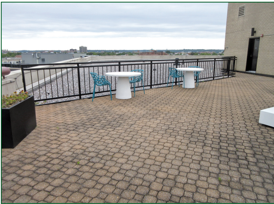
Figure 6. Pavers come in all shapes, sizes, and materials, and they are a common choice for use as walking surfaces at rooftop amenity spaces.
