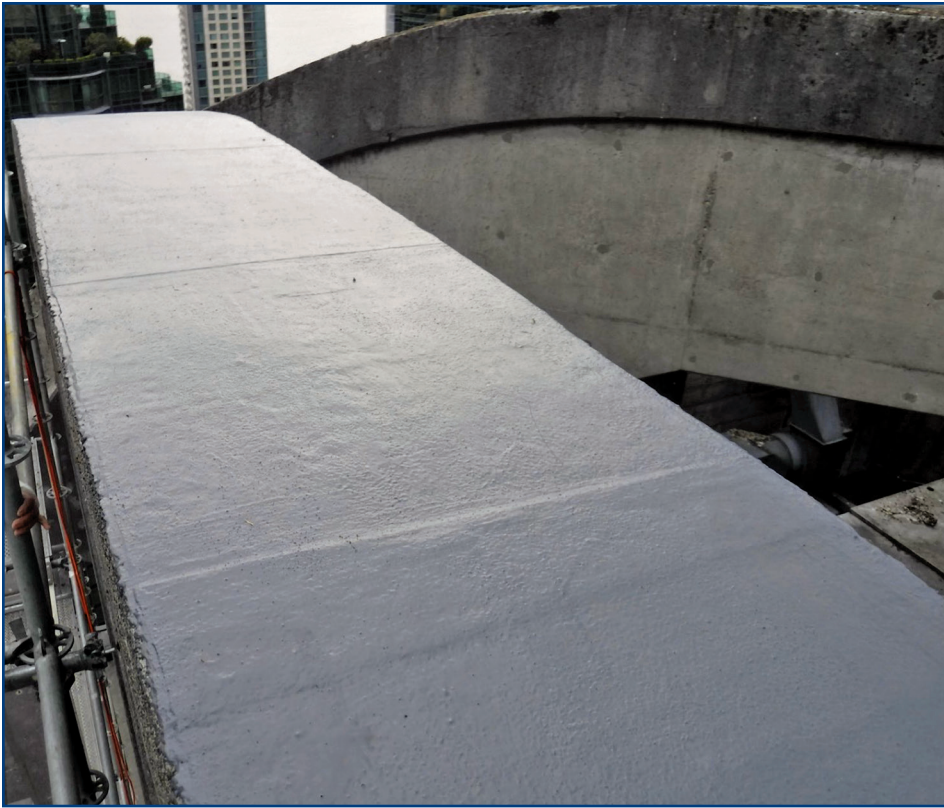
Figure 6. The horizontal tops of the concrete core and the cable enclosures were finished with a colored coating of polymethyl-methacrylate membrane.
