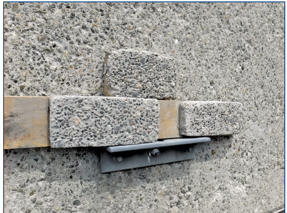
Figure 7. Careful selection of color additives and aggregate types produced a mixture design that was compatible with the existing concrete.
