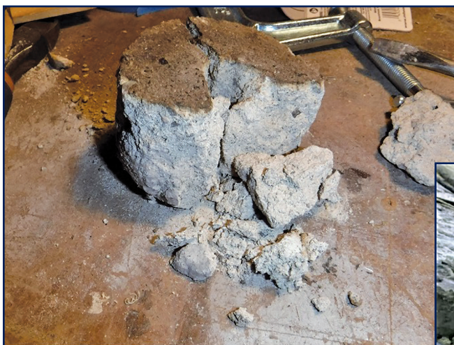
Figure 9. Core sample of a Nailcode topping course. It is highly recommended that this material be tested for asbestos as part of due diligence (during evaluation or design).
