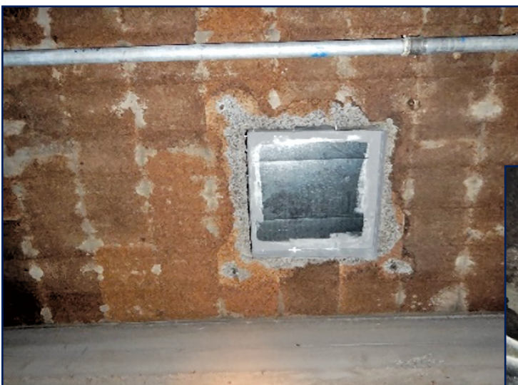
Figure 4. Note the bleed-through of concrete at regular intervals in the cork. At this subsequent rough opening, the "speckled" Haydite (shale aggregate here) is evident in the exposed section.
