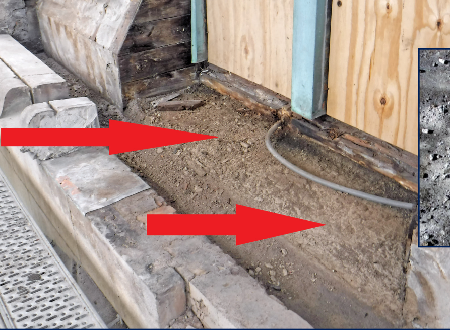
Figure 6. Nailcode topping extending from a gutter system that transitioned to flat-seam copper at the apron of window dormers. Wet material was encountered at these locations, prompting asbestos abatement and localized repairs.
