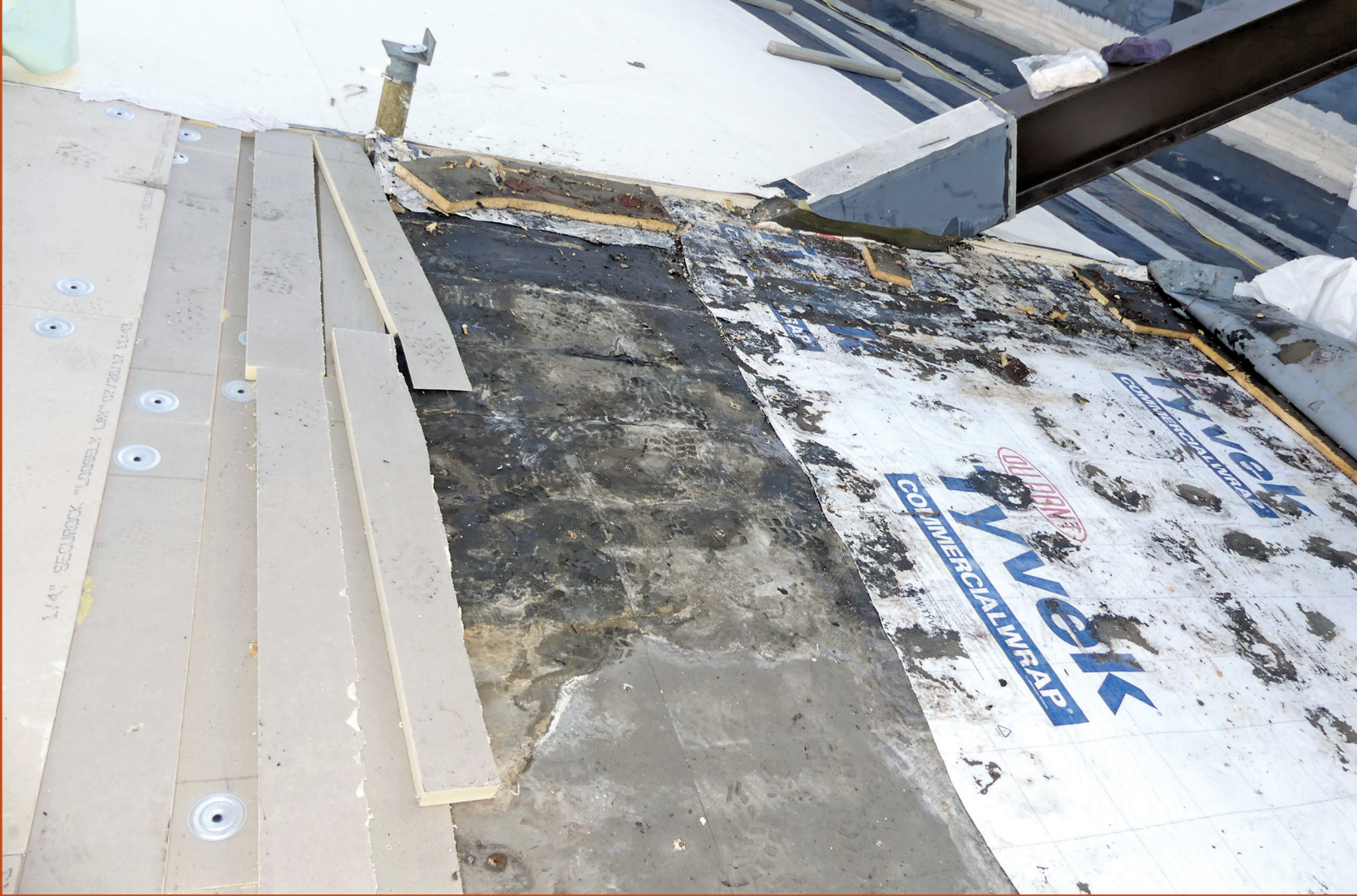
Figure 11. Tear-off in progress at lower dome. Note the signs of moisture on the existing insulation.
