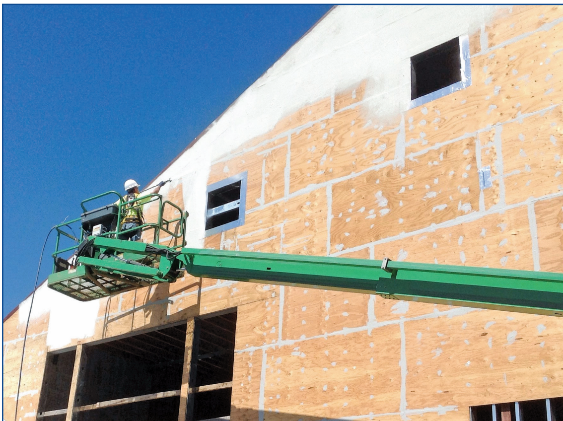
Figure 10. Spray application of liquid-applied weather-resistant barrier was used on the A to Z Wineworks project in Newburg, Ore.
