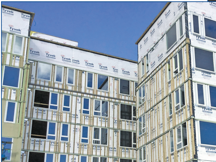
Figure 5. Rainscreen furring and flashings installed at the Tony Lee Apartments-Lake City Family Housing in Seattle, Wash.
