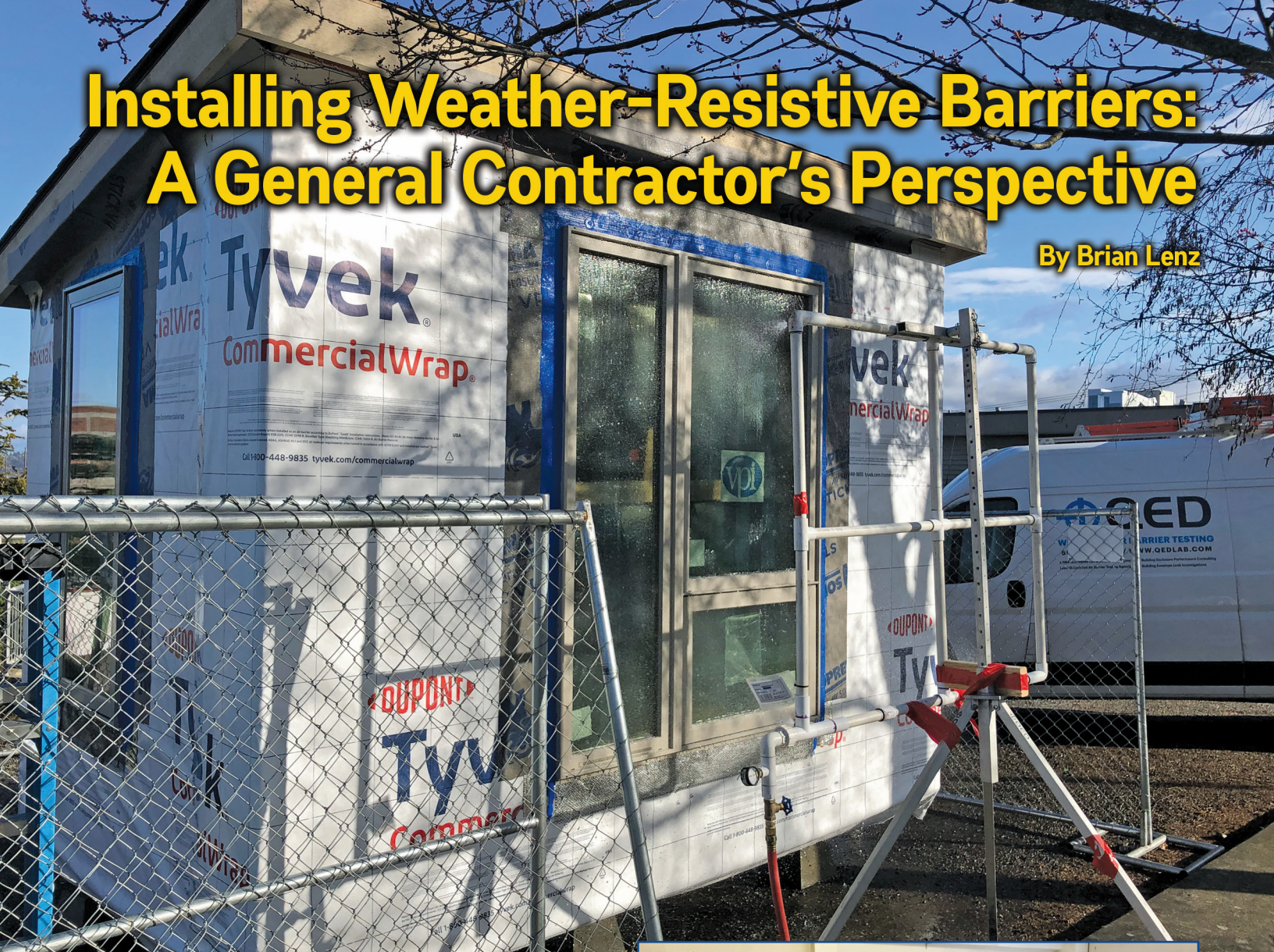
Figure 1. Walsh Construction Co. typically builds project mock-ups as “tiny houses,” which are subsequently donated to the Low-Income Housing Institute, one of Walsh’s longtime nonprofit clients. (Window testing performed by QED Lab, Troutdale, Ore.)
