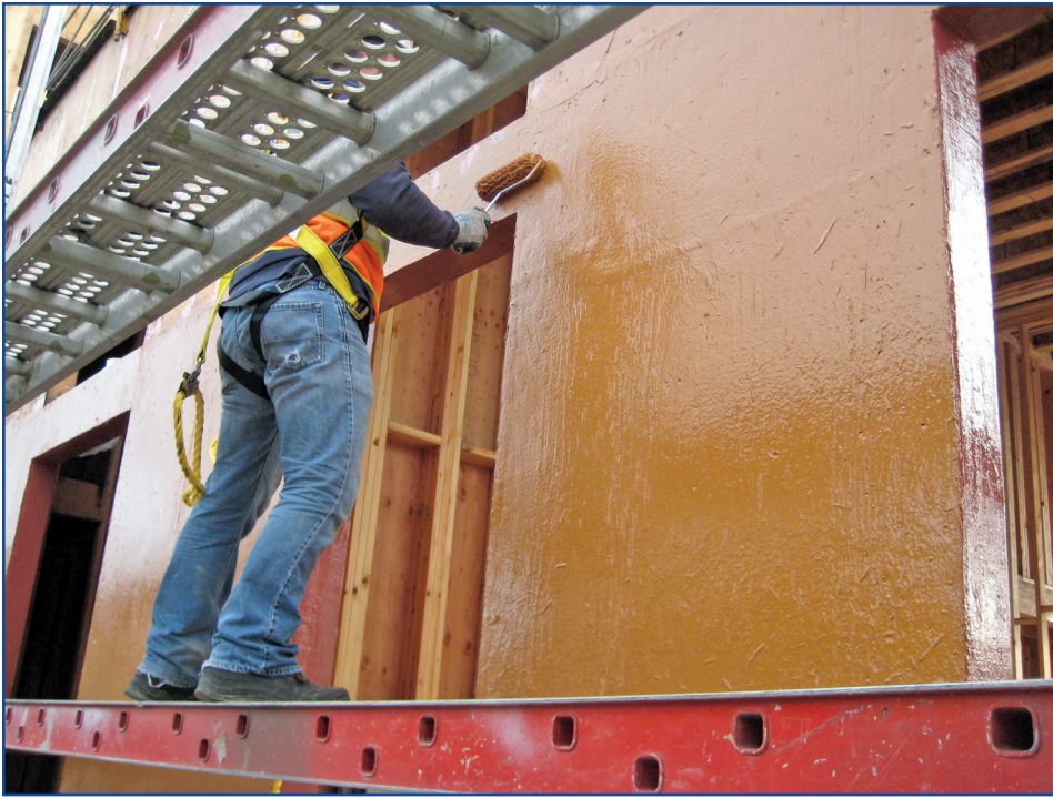
Figure 11. An installer using a roller to apply a liquid-applied weather-resistant barrier with liquid flashing into the door and window rough openings.
