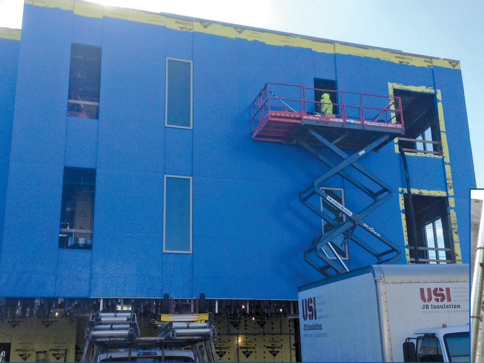
Figure 8. The Asian Health and Service Center in Portland, Ore., with a liquid-applied weather-resistant barrier.
