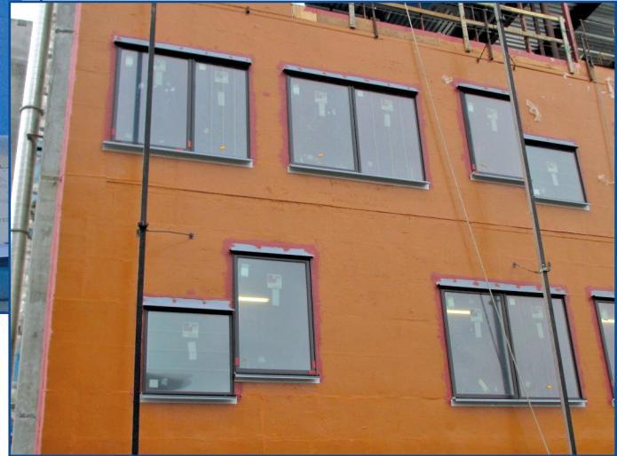
Figure 9. The building enclosure for the Greenfire Campus in Seattle, Wash., includes a liquid-applied weather-resistant barrier and liquid flashing over sheet metal head flashings.
