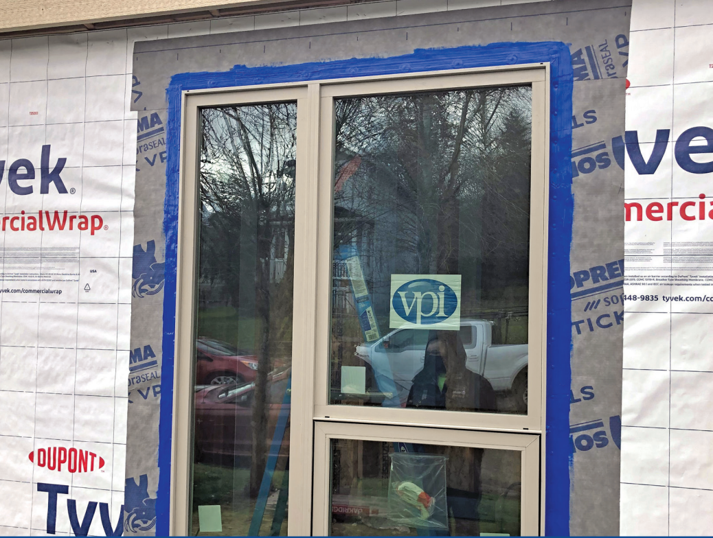
Figure 12. An example of a “hybrid” installation, which uses mechanically fastened and self-adhered weather-resistive barriers as well as liquid flashing applied over vinyl window flanges.
