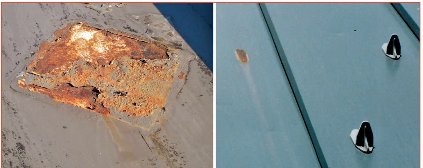
Figure 10. Examples of adhesive bond to paint. Even if the adhesive does not fail, the paint adhesion might, leading to corrosion.
