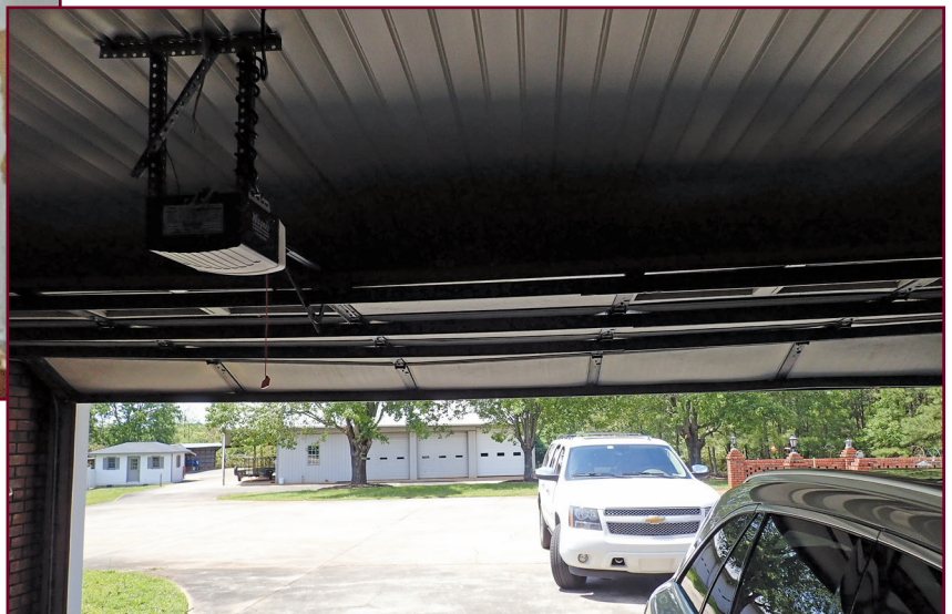
Figure 11. View of damaged aluminum garage door framing and panels.
