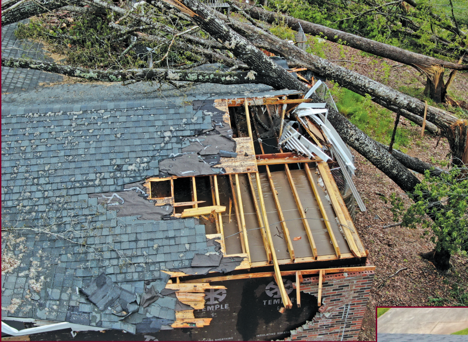
Figure 4. View of displaced wood roof framing, roof decking, and roof covering.
