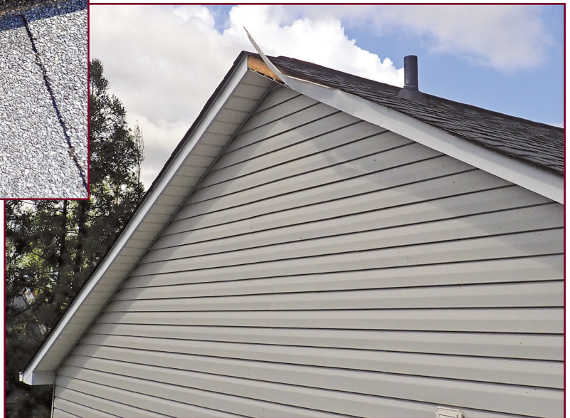
Figure 7. View of displaced metal rake trim.
