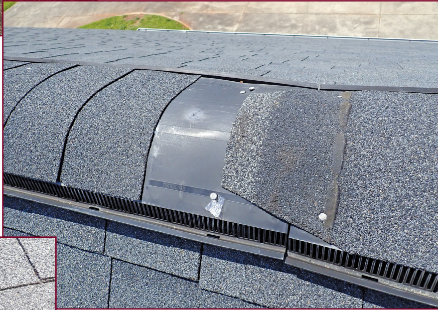
Figure 5. View of displaced shingles at ridge.
