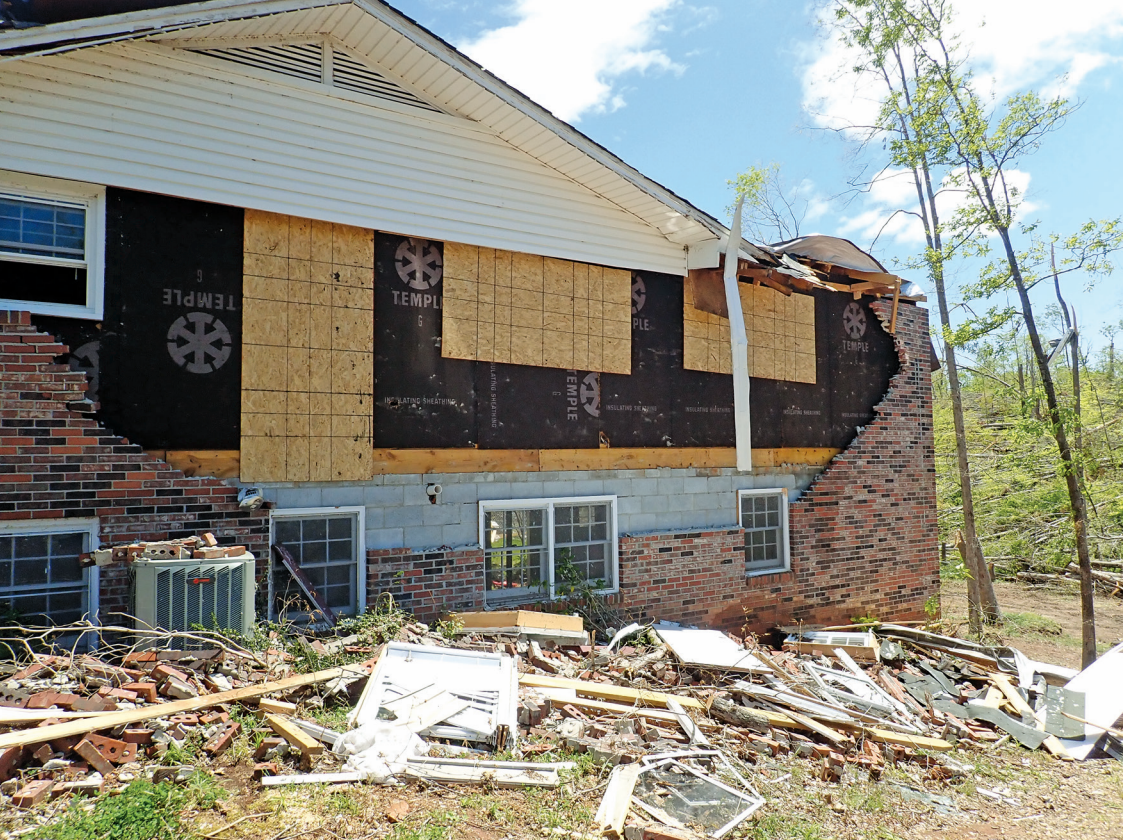
Figure 8. Partial displacement of brick veneer cladding. OSB panels cover window and door openings.
