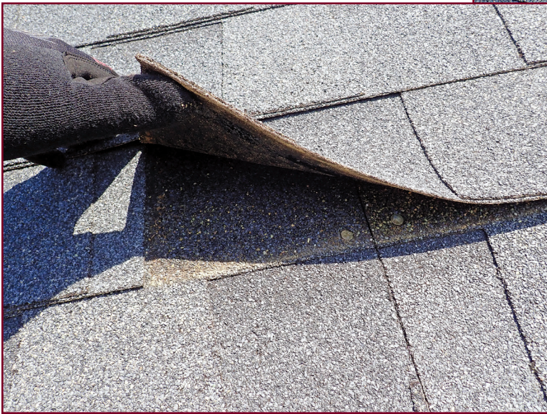
Figure 6. View of unadhered laminated composition shingle.
