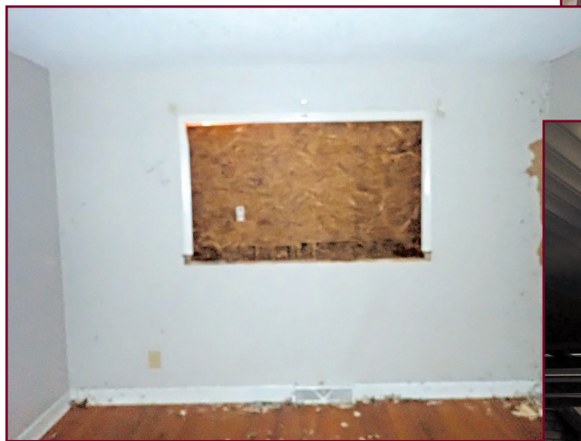
Figure 10. View of complete displacement of window from rough opening.
