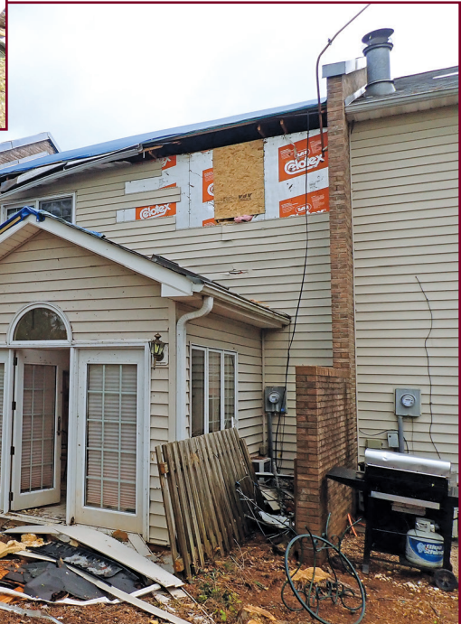
Figure 9. View of displaced vinyl siding.
