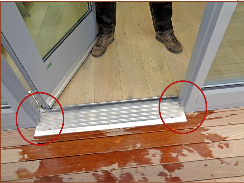
Figure 4. Discontinuity at the low-profile threshold of storefront assembly. The adjacent storefront subsill and frame do not extend under the doorframe area.
