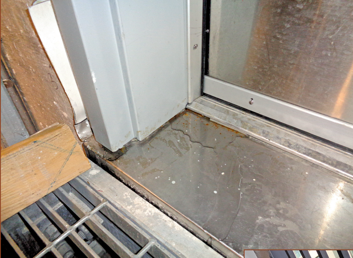
Figure 8. Water leakage at a hollow metal door's jamb-to-sill corner.
