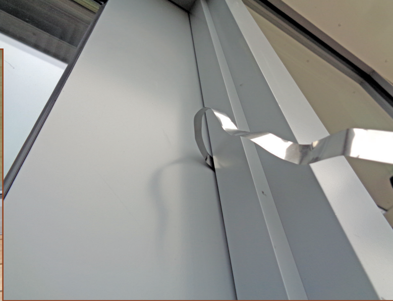
Figure 5. Metal feeler gage extended between the doorframe and operable storefront door to show that gaskets are not compressed.
