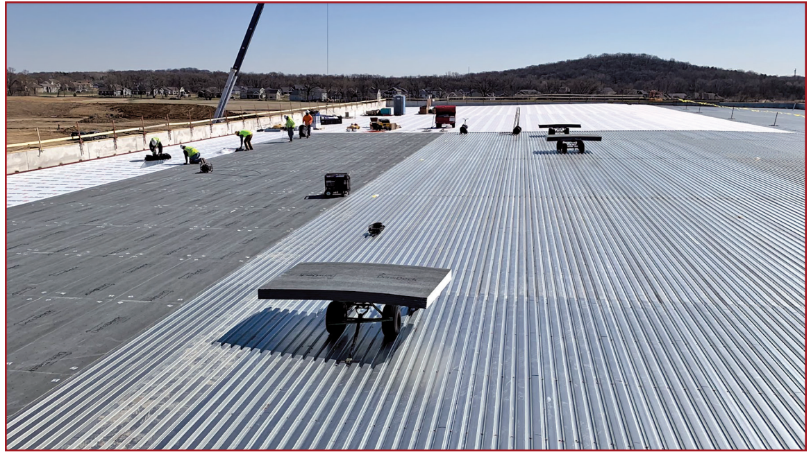
Figure 5. Installation of a gypsum-based board over a metal deck. The ability for workers to walk on this surface without doing harm to the rigid board is critical to the long-term success of the roof system.
