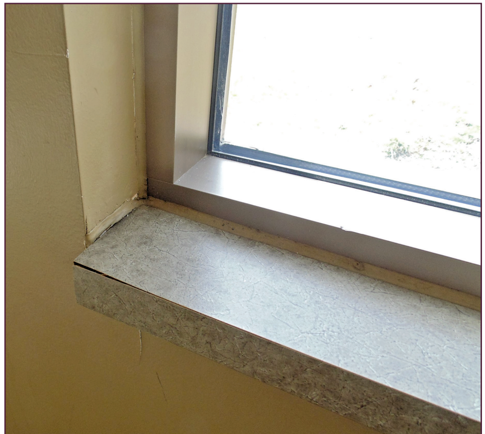
Figure 1. Visible moisture damage of the plastic laminate sills. Photo courtesy of Inspec.
