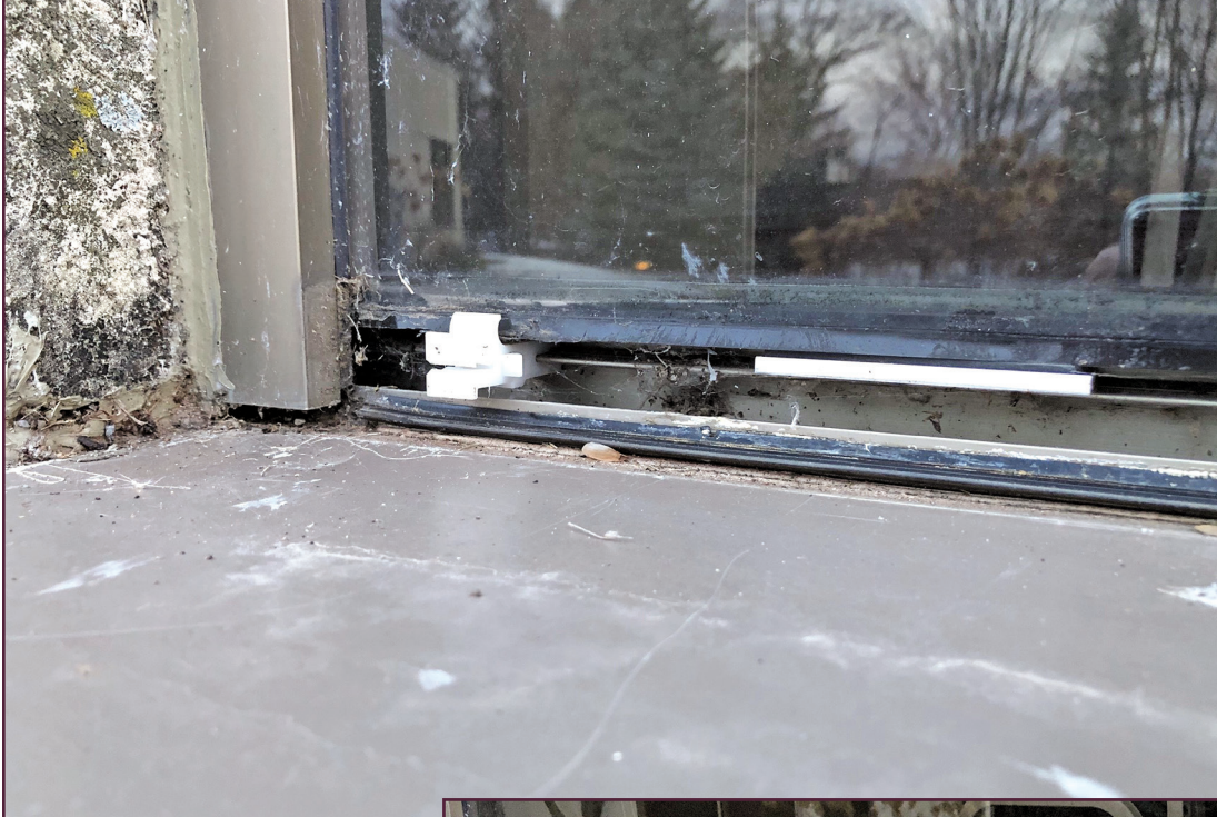
Figure 2. Plastic clips secured the aluminum to the glazing gaskets, allowing movement and water entry. Photo courtesy of Inspec.
