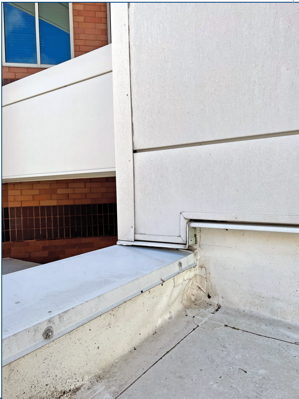
Figure 5. A thermoplastic polyolefin-clad parapet wall transition to exterior insulation and finish system condition.
