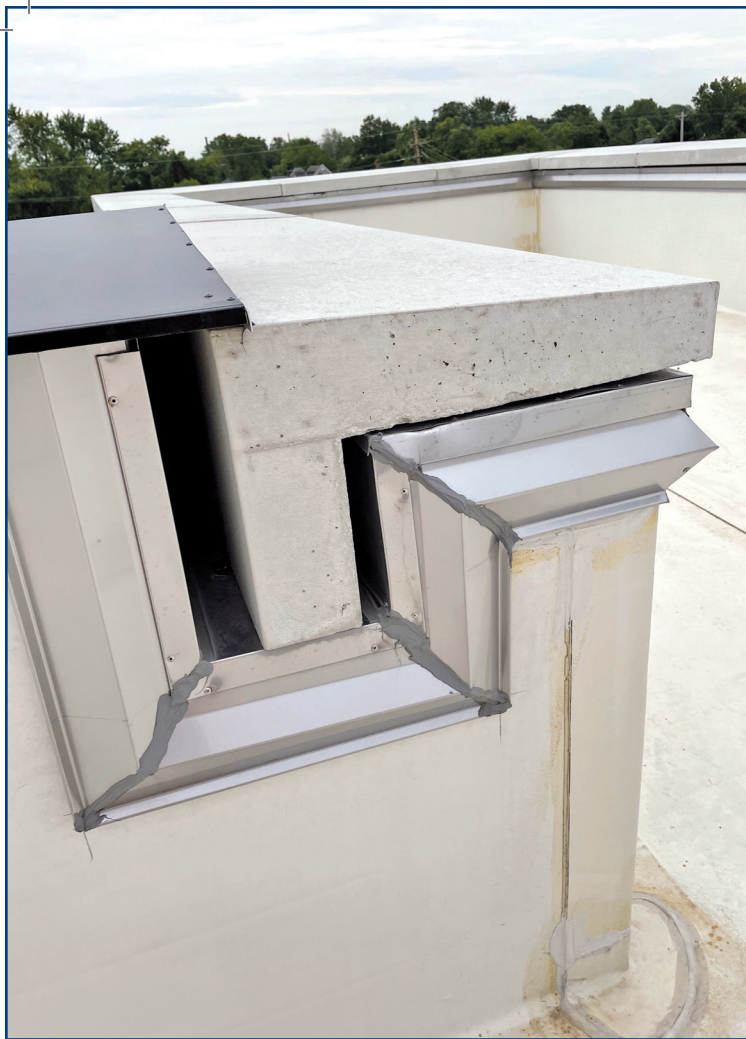
Figure 12. An inside corner of a parapet wall clad with white ethylene propylene diene terpolymer to stone and sheet metal coping termination detail condition.
