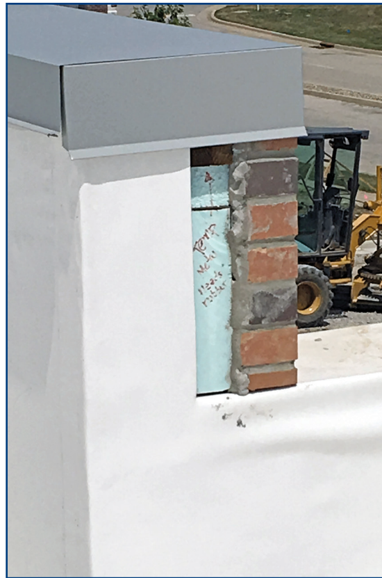
Figure 8. A thermoplastic polyolefin-clad parapet wall transition to exterior face brick veneer condition.
