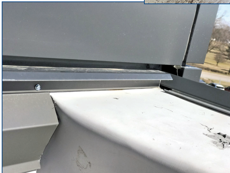
Figure 4. A thermoplastic polyolefin-clad parapet wall transition to an aluminum composite material condition.
