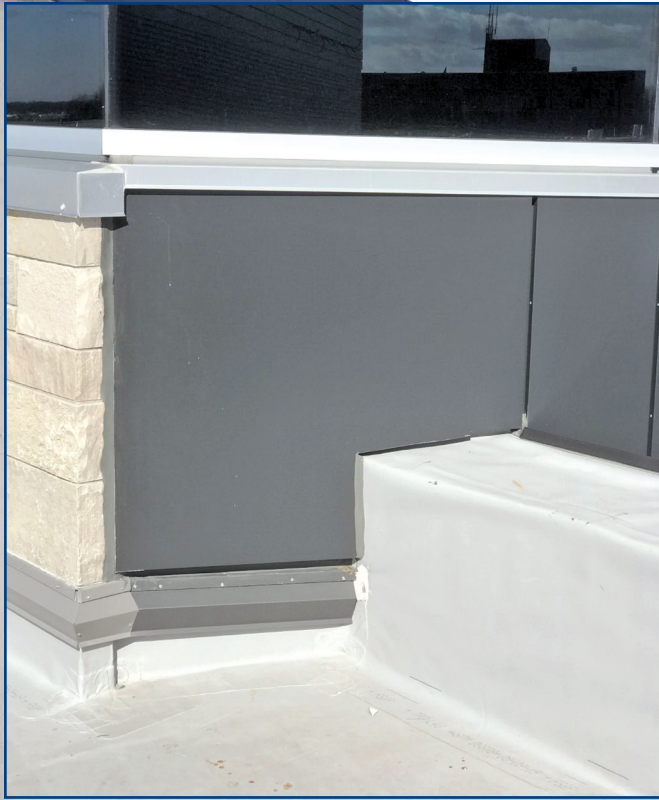
Figure 2. A thermoplastic polyolefin-clad parapet wall transition to a field-trimmed aluminum composite material condition.
