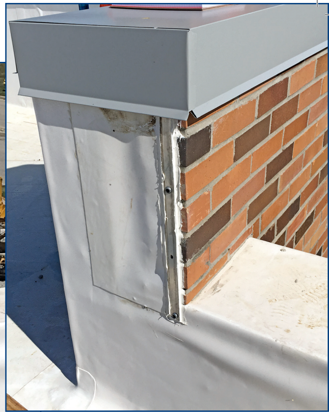
Figure 9. A thermoplastic polyolefin-clad parapet wall transition to exterior face brick veneer condition.
