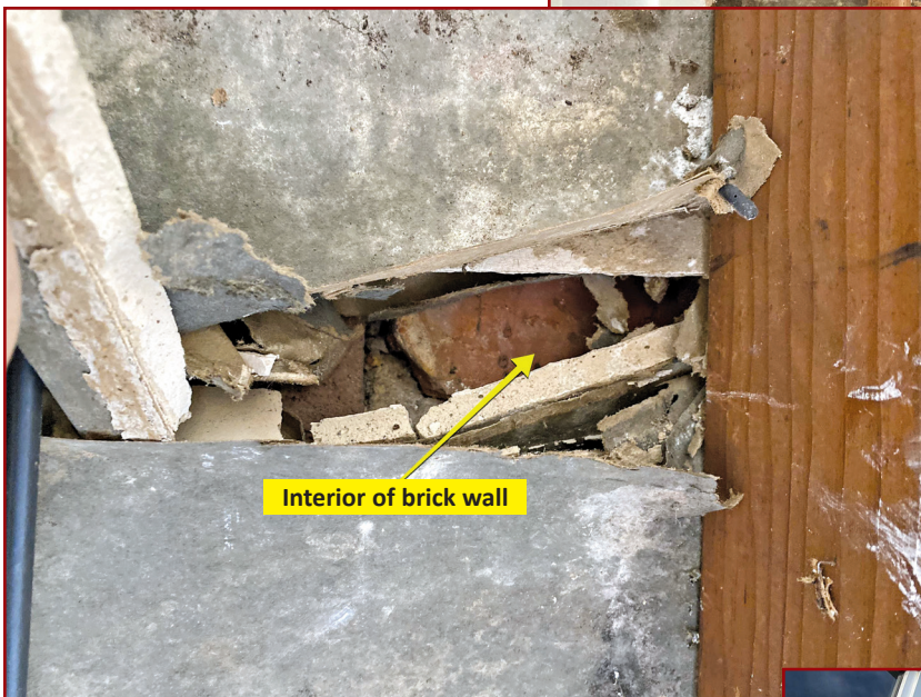
Figure 6. The weather barrier easily crumbled due to excessive moisture saturation.
