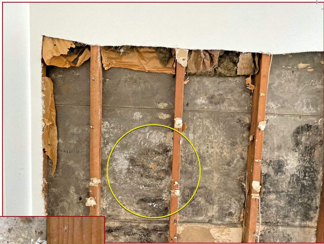
Figure 5. The interior of the leak area with organic growth on the weather barrier.
