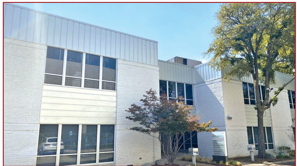
Figure 1. This masonry facade was retrofitted with continuous metal panels at the interstitial space between the roofline and the second-story ceiling.
