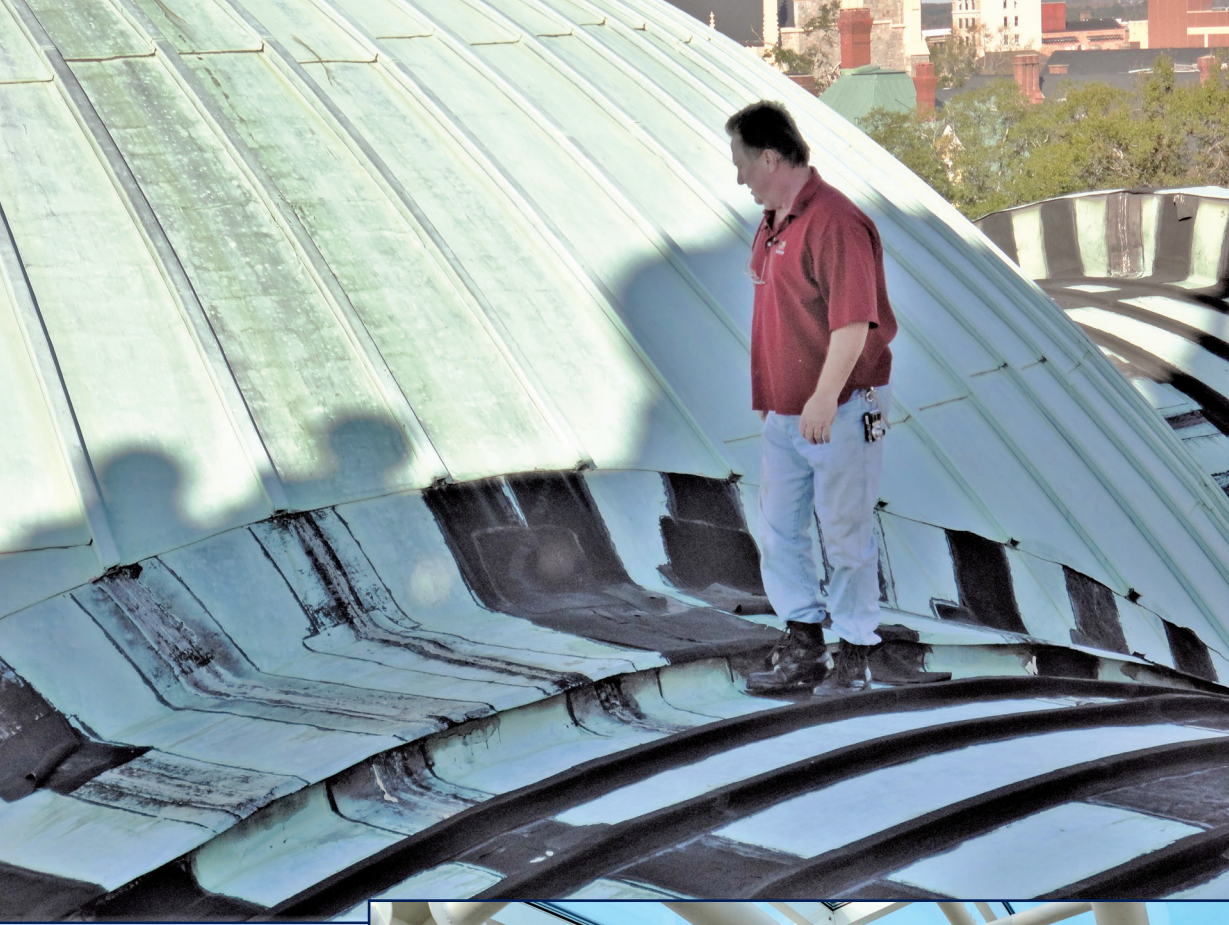
Figure 4. This church dome and the adjoining bell tower were experiencing chronic leakage even though ethylene propylene diene monomer (EPDM) and Neoprene rubber had been used to patch the seams and panel ends. Whatever repairs would have been appropriate on this copper would not have involved rubber patches.
