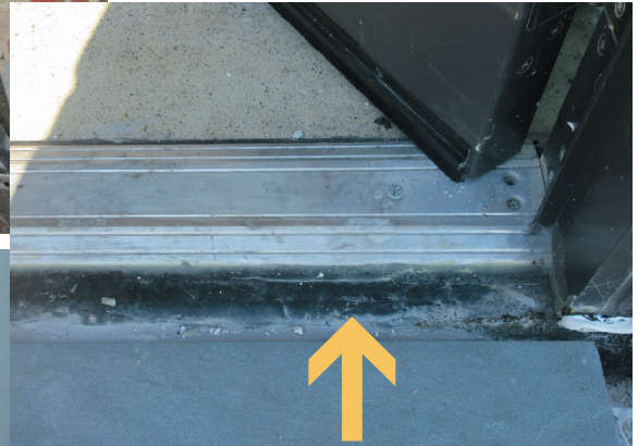
Figure 7. Exposed terrace waterproofing outboard of threshold is not designed for exposure to ultraviolet light and direct foot traffic.
