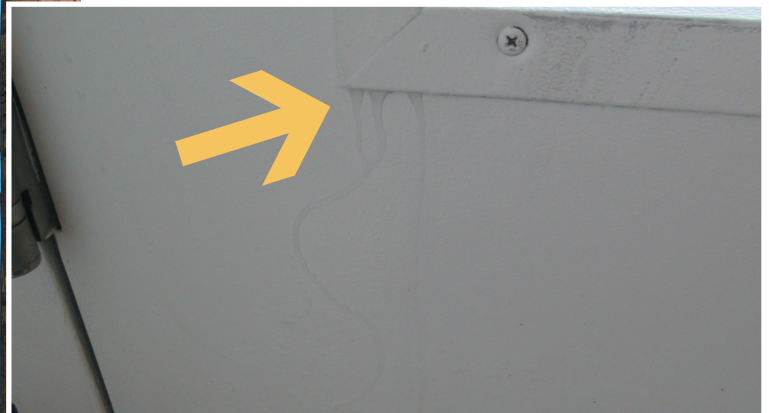
Figure 3. Active leak at the lower corner of a glazing unit installed within a terrace door assembly.
