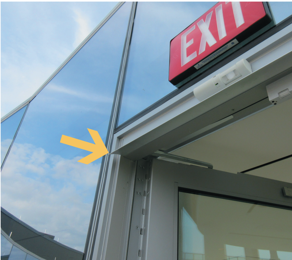
Figure 10. Drip edge installed at the head of a doorframe located at a roof-level terrace.
