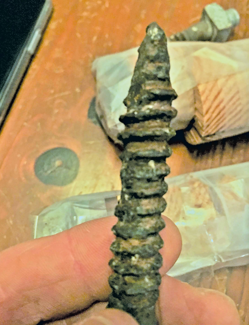
Figure 10. The hanger screw removed from upper left corner (see Fig. 5) of the lower balcony had severely corroded threads. Photo: Thomas H. Lutge, SE ( http://www.quakestructural.com ).
