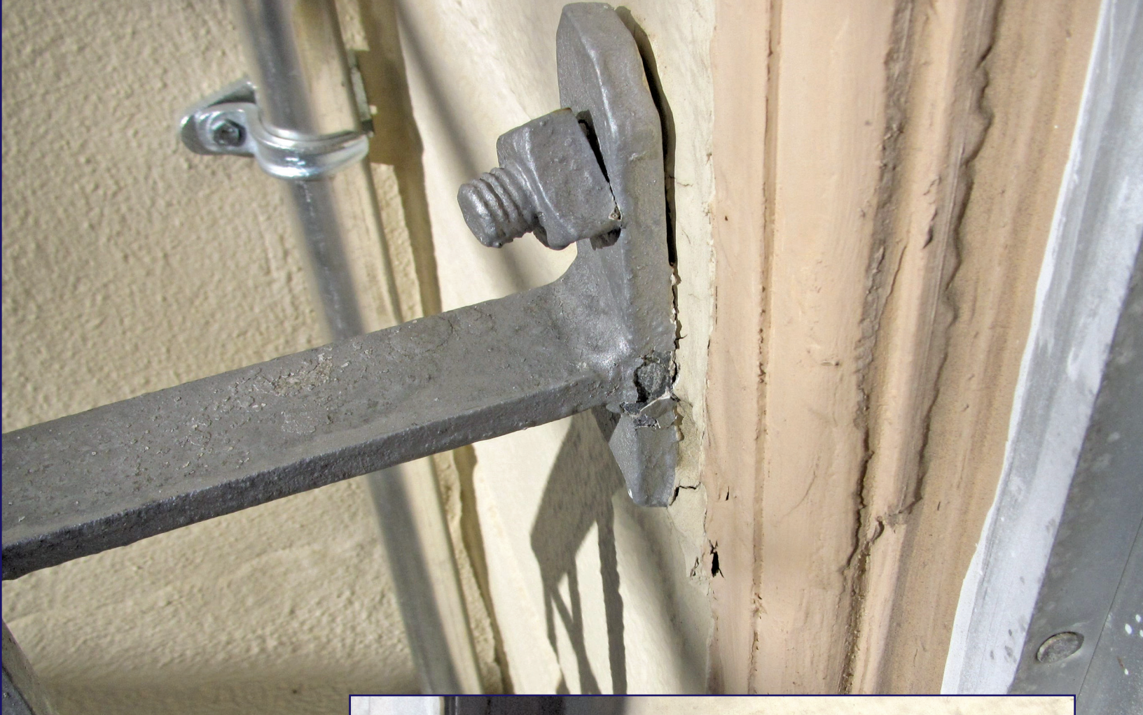
Figure 5. The lower balcony was attached at the upper corners with 4-in.-long, ½-in.-diameter hanger screws. This fastener exhibits evidence of an axial prying action and withdrawal, as compared with the opposite hanger screw shown in Fig. 6. Note: 1 in. = 25.4 mm.
