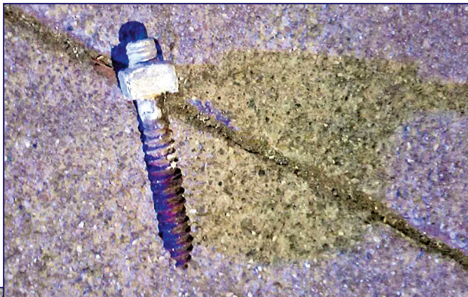
Figure 7. San Francisco Police Department photograph of a failed hanger screw from the night of the balcony collapse.
