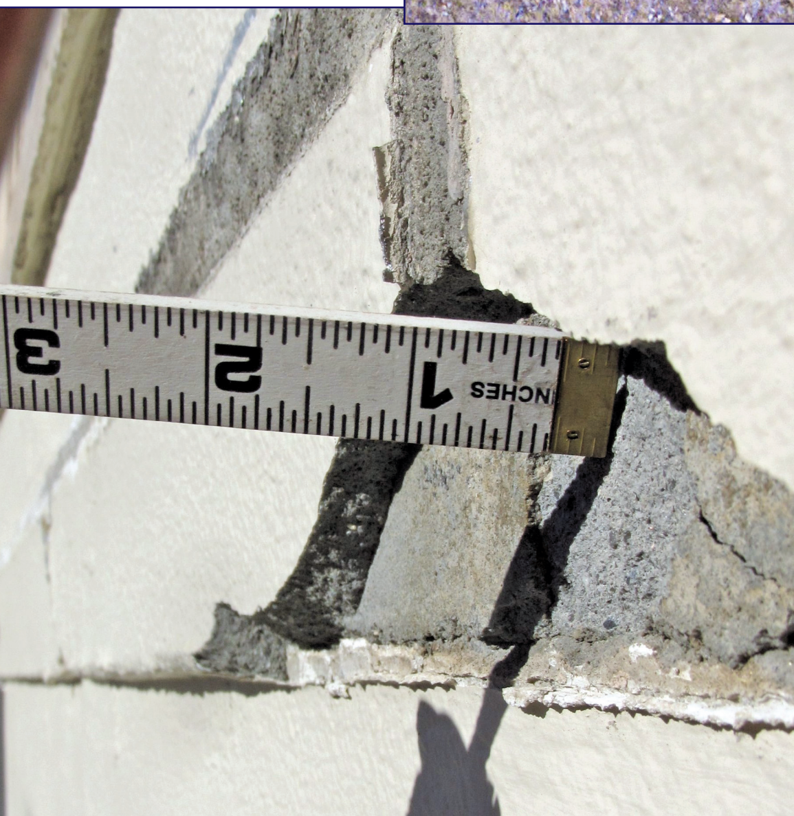
Figure 8. Damage from the failed wood screw shown in Fig. 4 to the 1/4-in.-thick layer of decorative plaster cement applied for aesthetic relief atop an underlying 3/4-in.-thick stucco cladding assembly. Note: 1 in. = 25.4 mm.
