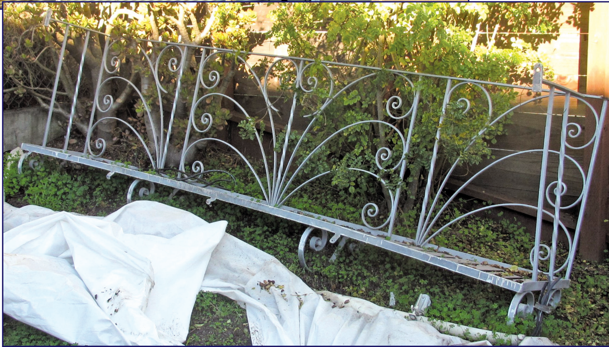
Figure 3. After its sudden collapse, the failed balcony was stored in the backyard for expert inspection.
