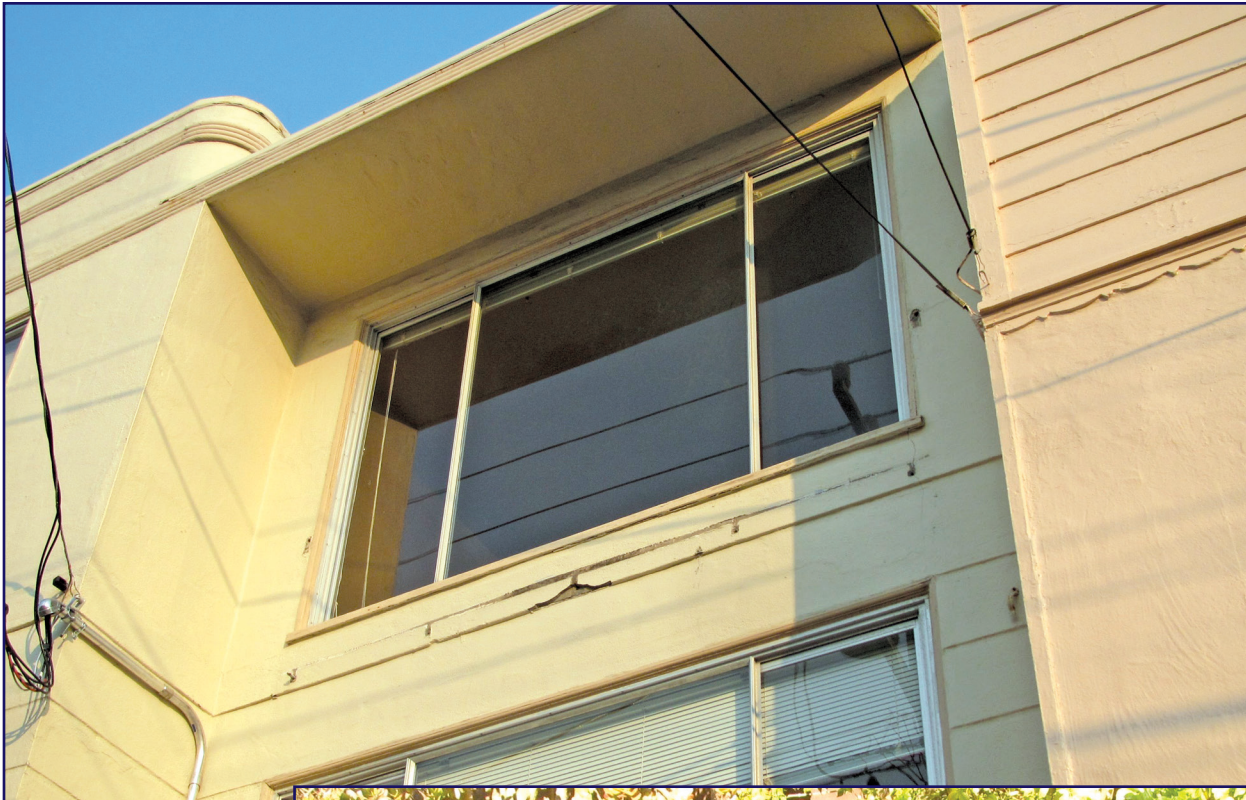
Figure 2. Window at the upper apartment after the wrought iron balcony collapsed. The collapsed balcony was identical to the one shown in Fig. 1.
