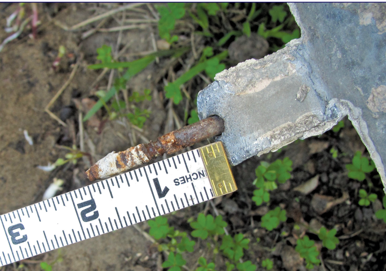
Figure 4. The bottom edge of the failed balcony was secured to the stucco-clad wall with five wood screws. Note: 1 in. = 25.4 mm.
