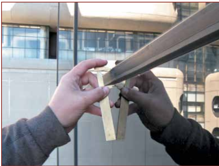
Figure 3. Out-of-plane glass across a floor line in an early curtainwall.
