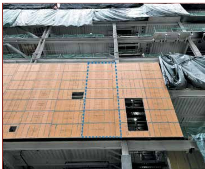
Figure 5. Large-format panels on a commercial high-rise building. Panel size is indicated by the blue dashed lines.
