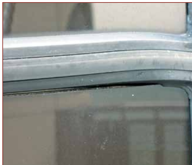
Figure 4. Dislodged glass below a floor line in an early curtainwall.
