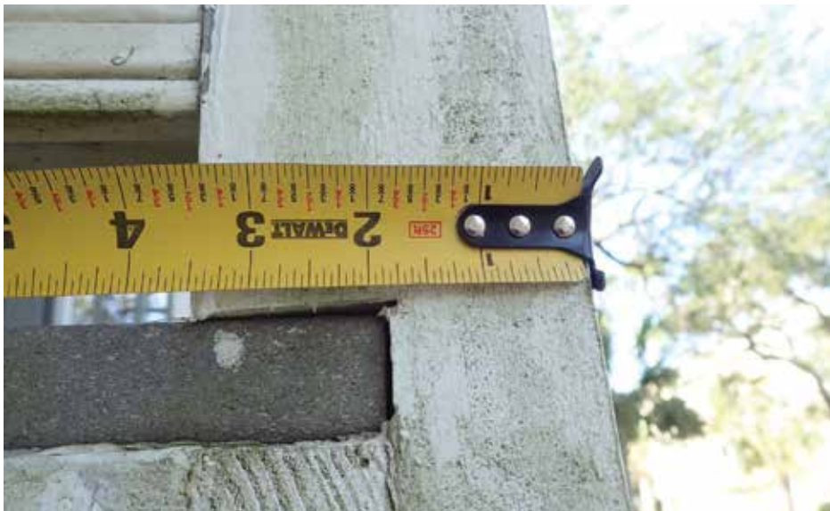
Figure 5. Notching one-half of a 4- × 4-in. wood guardrail post violates the building code. Note: 1 in. = 25.4 mm.
