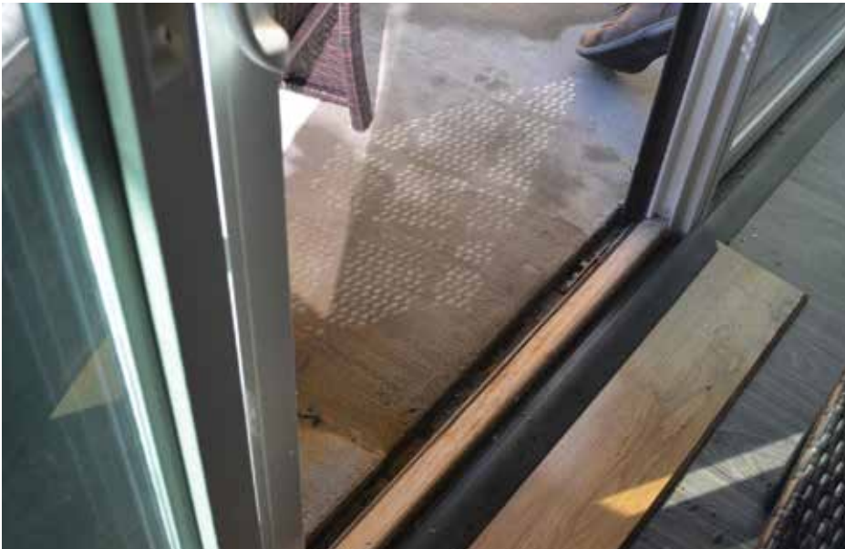
Figure 12. Setting the balcony door threshold below the concrete balcony surface is asking for trouble.
