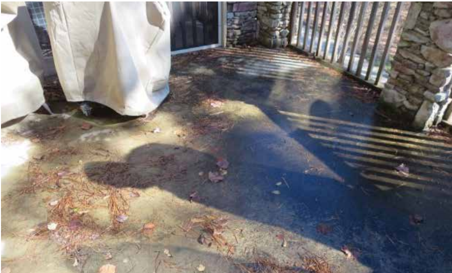
Figure 2. Ponded water on a balcony surface.
