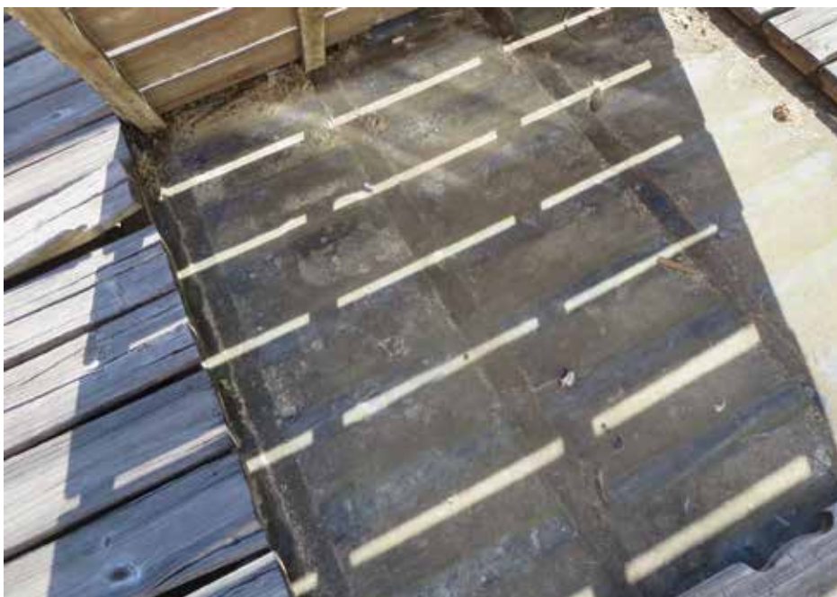
Figure 6. Wood deck “sleepers” installed over an ethylene propylene diene terpolymer (EPDM) membrane.
