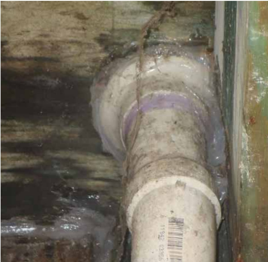
Figure 13. A retrofit drain installed in a balcony with slope/drainage issues will have limited success unless water is directed to it via proper design and construction.
