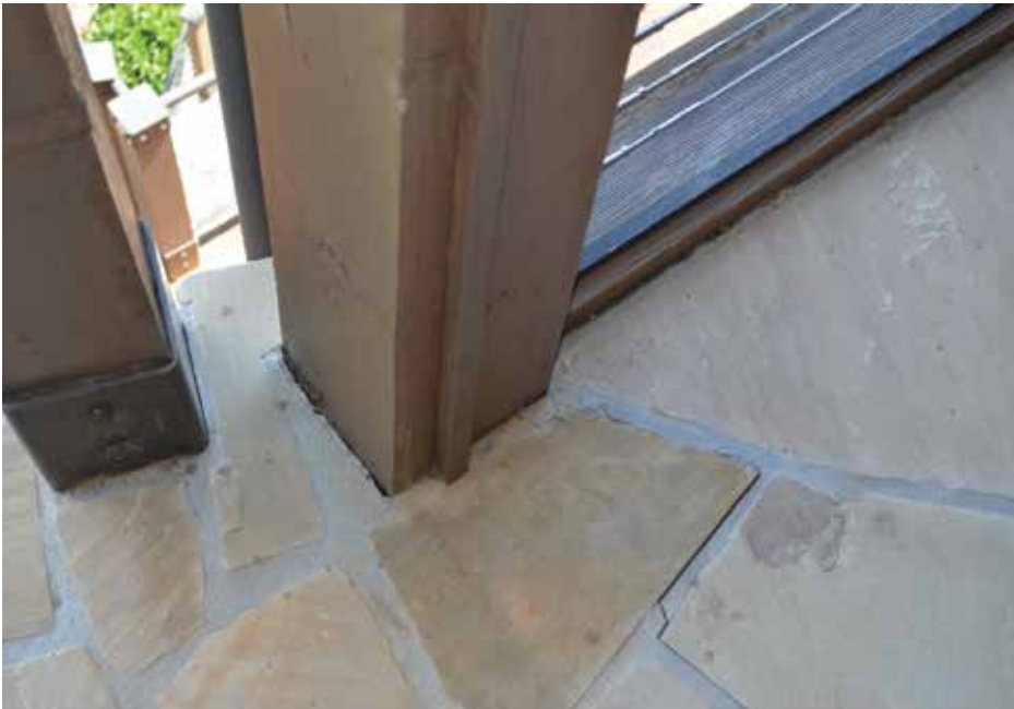
Figure 7. Large wood columns interrupt the waterproofing at a balcony edge.
