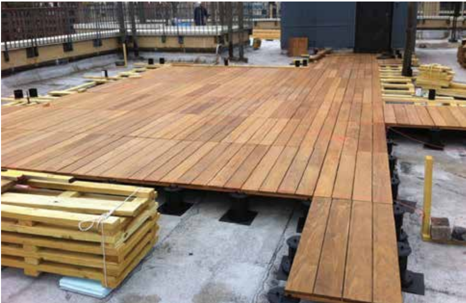
Figure 9. A pedestal system serves to separate the waterproofed surface from the pedestrian walking surface.
