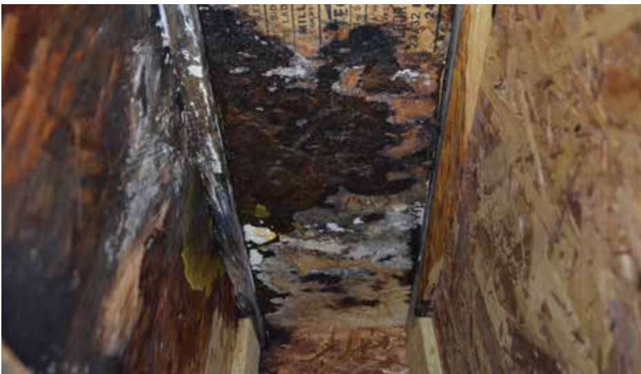
Figure 8. Significant framing damage below the balcony shown in Fig. 7.
