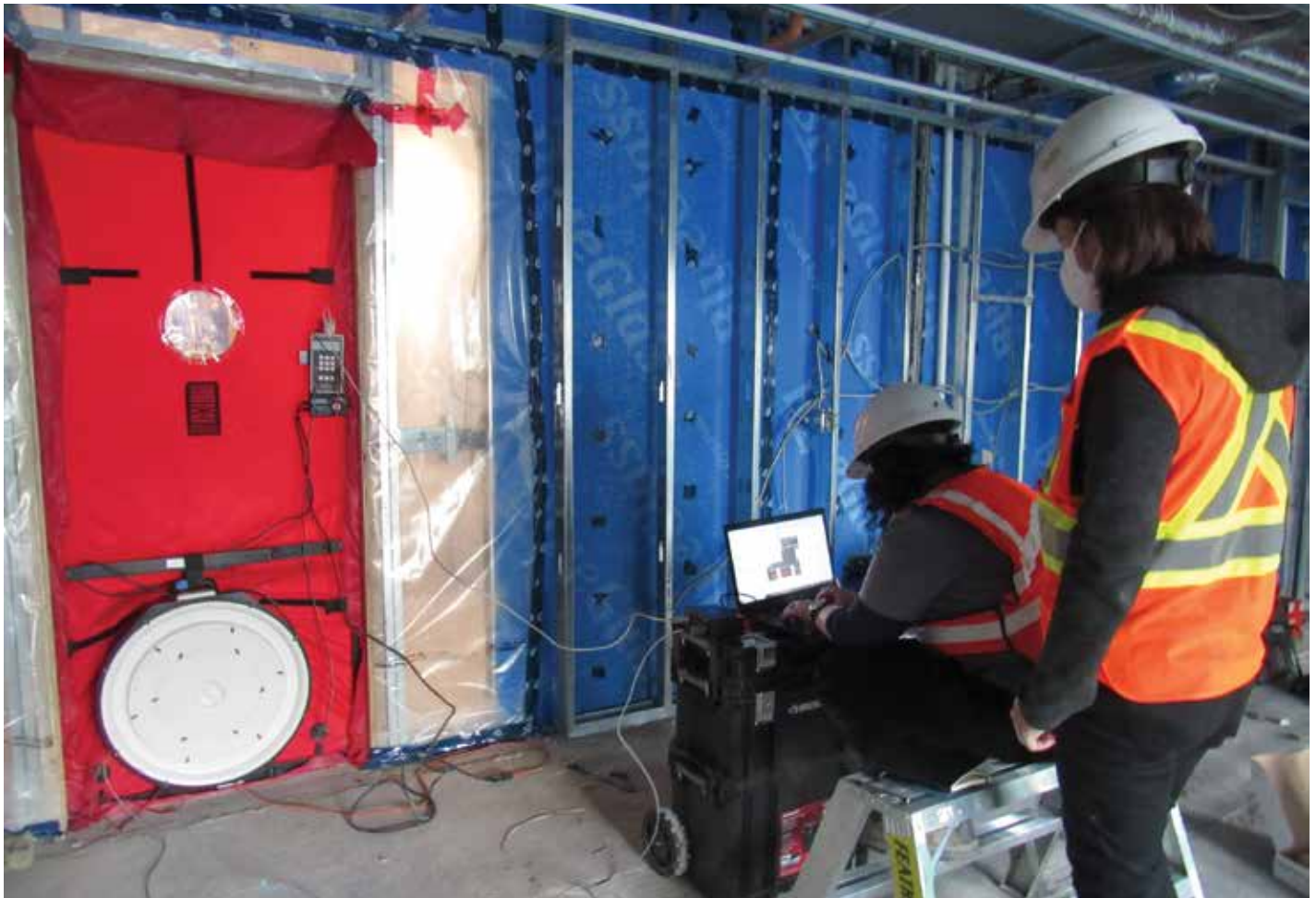
Figure 1. Technicians running a series of blower doors connected through a central hub.
