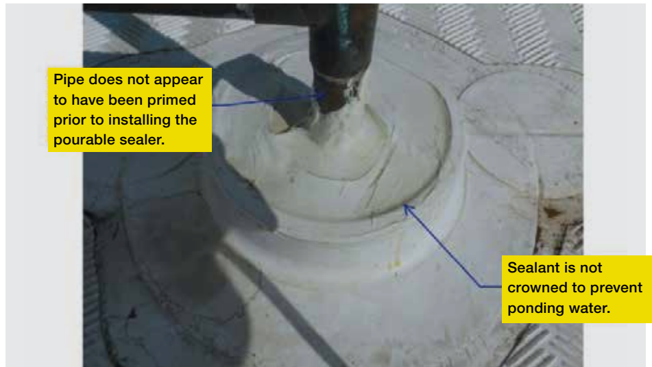
Figure 8. Example of incorrectly installed sealant-pocket flashing. The sealant in the pan is not crowned, and the contractor did not prime the thermoplastic olefin membrane flashing or the pipe before installing the pourable sealer.
