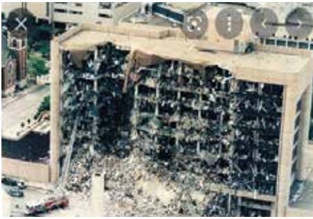
Figure 4. The Alfred P. Murrah Federal Building in Oklahoma City, Oklahoma, after it was bombed.
