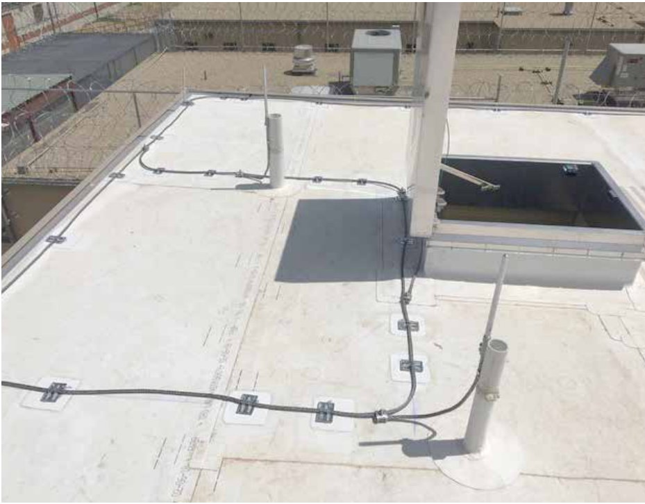
Figure 4. Multiple paths are created with the use of properly placed strike termination devices and conductors.
