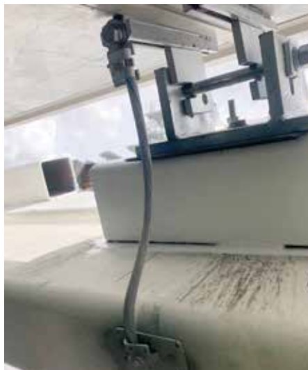
Figure 9. Early coordination enabled the lightning protection system to be concealed; conductors are internal to the structure.
