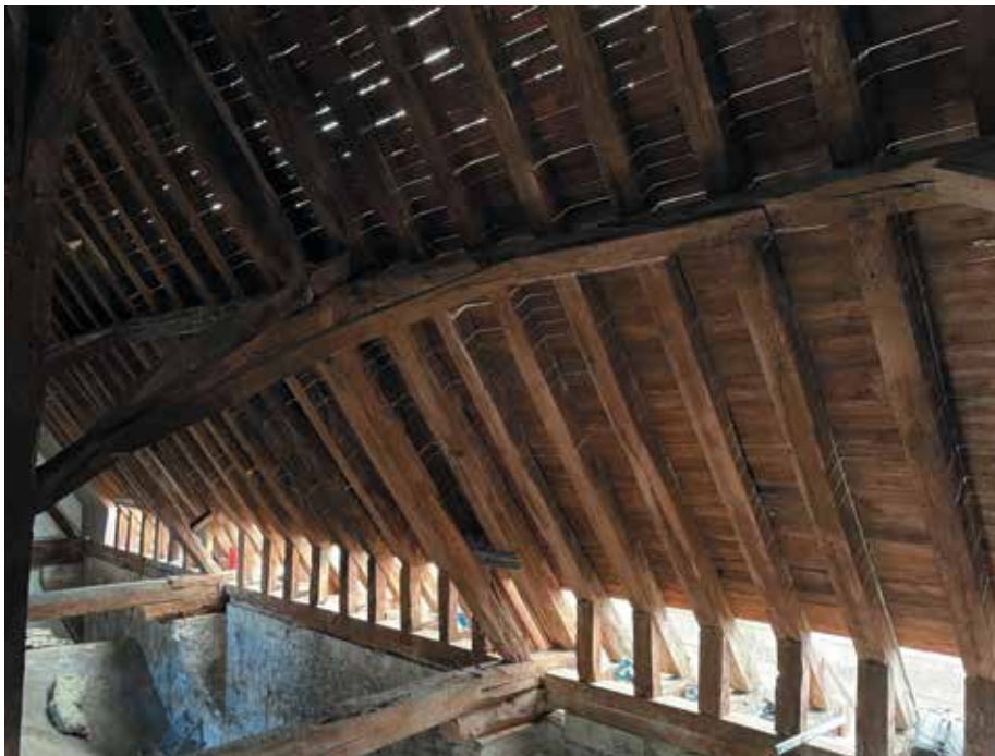
Figure 5. Medieval timber supporting the nave roof; with the external copper removed, daylight shines through penny gaps between sheathing boards.
