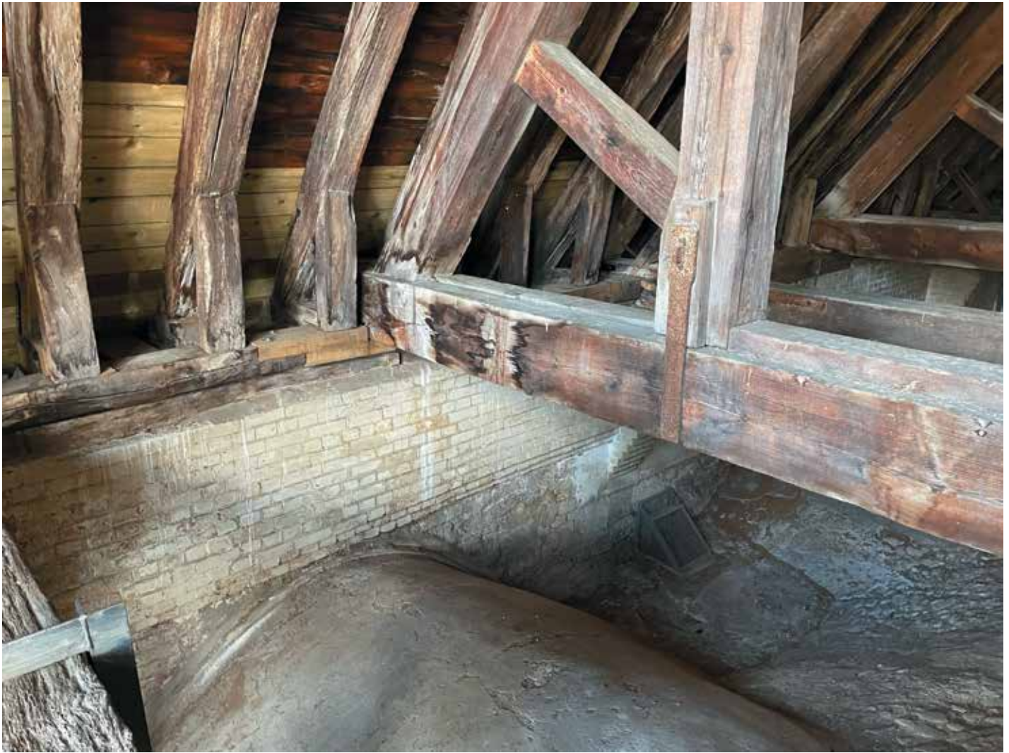
Figure 4. Rainwater staining of timber structure, including a replaced wall plate.
