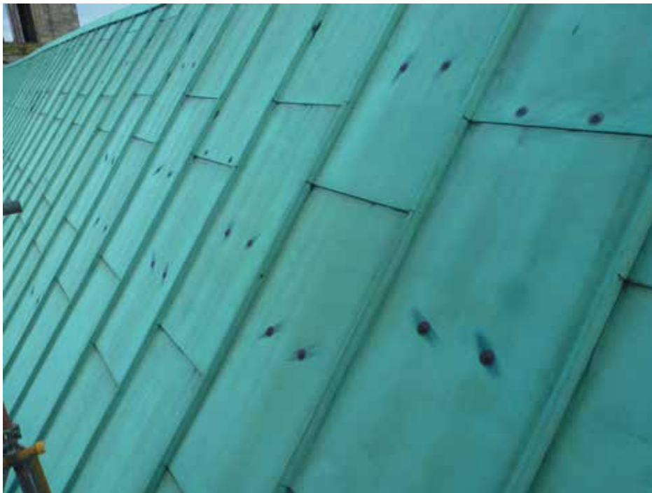
Figure 3. The 1949 copper roofing with additional fasteners to reduce uplift and splitting.
