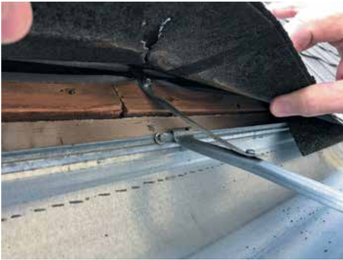
Figure 1. Example of a critical eave where drip edge was not installed even though it is the minimum required standard. Ethical decision-making means doing what's right for the client even when no one is looking.
