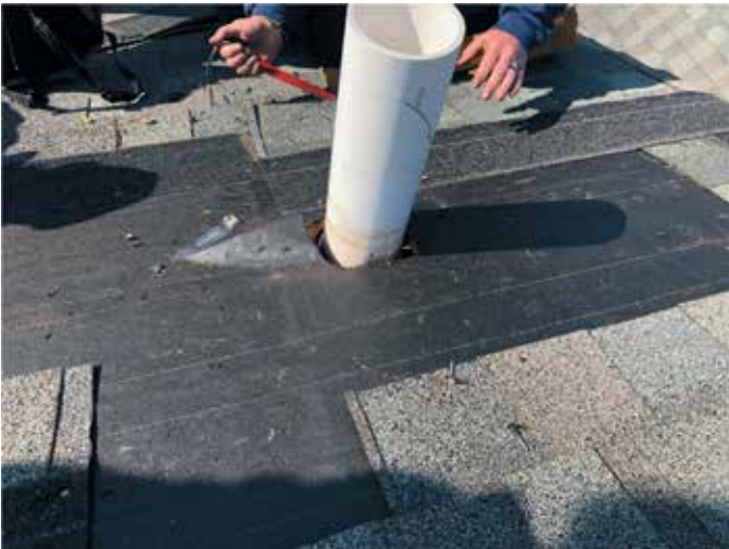
Figure 3. This pipe penetration was never flashed per minimum required industry and manufacturer standards, resulting in persistent leaks that went undiagnosed by the original roofer in subsequent service calls for over three years.
