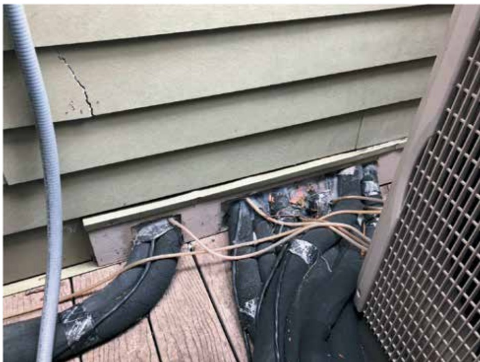
Figure 10. Improper wall penetrations and termination detailing resulting in substantial leaks into the space below.
