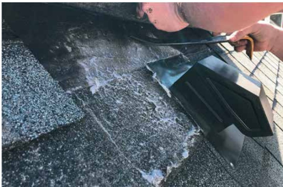
Figure 9. Dryer exhaust penetration through roof, unsealed and building up around penetration.
