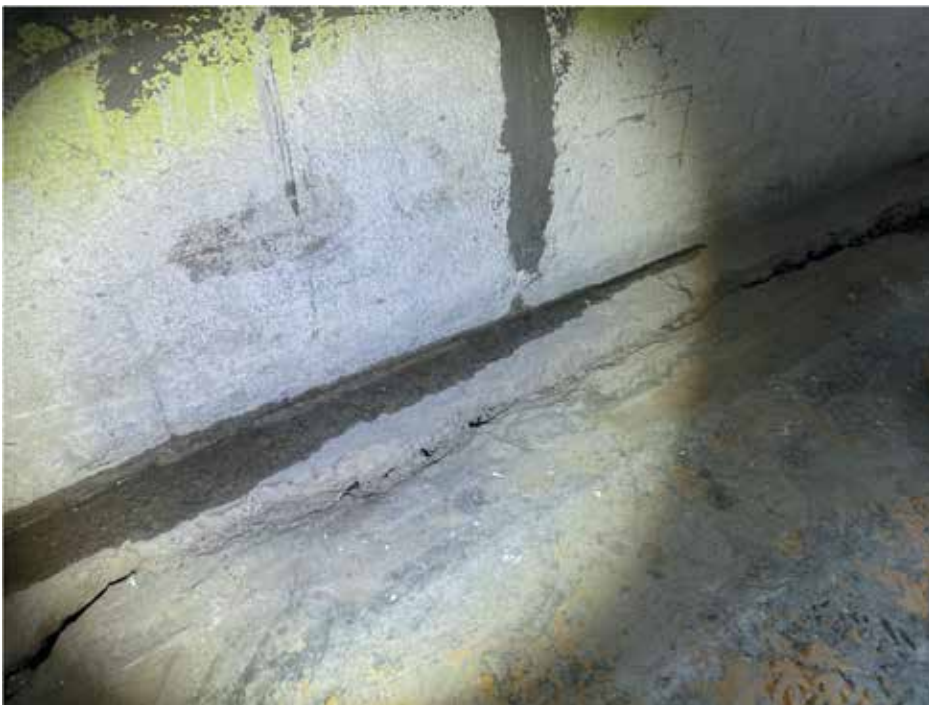
Figure 6. Moisture intrusion at masonry wall confirmed during testing.
