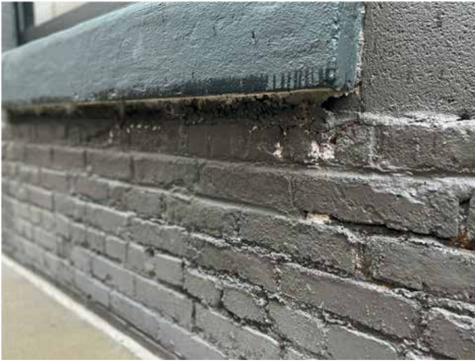
Figure 5. Evidence of moisture intrusion at masonry wall and numerous voids in the coating allowing water entry.
