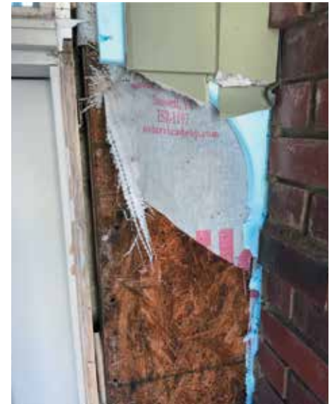
Figure 8. Improper weather-resistive barrier application and flashing sequence—active moisture intrusion and damage to substrate and water entry at doorway rough opening.
