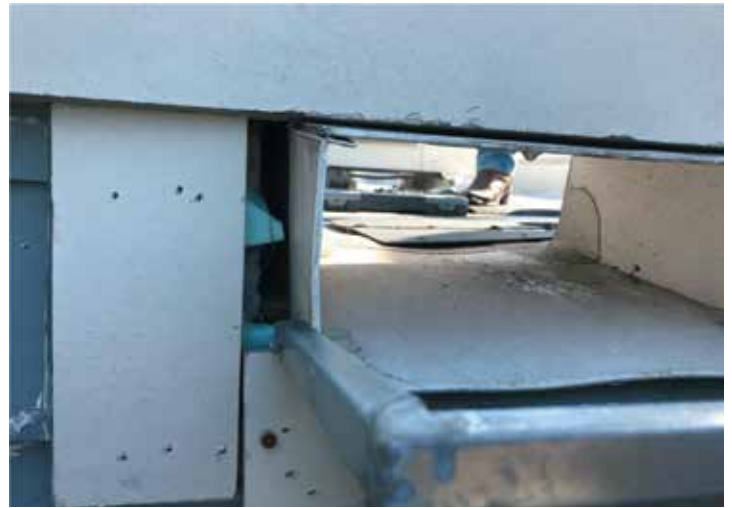
Figure 2. Example of improper terminations missed/ignored by all coordinating trades even though proper termination to prevent water entry is the minimum required standard. Ethical decision-making in this scenario means refusing to leave an at-risk area incomplete in the interest of the client and occupants of the building.
