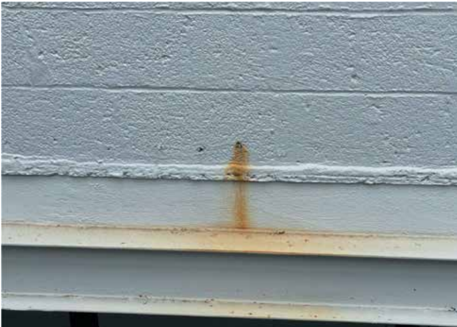
Figure 7. Evidence of moisture intrusion at masonry wall shown as rust escaping a wall void.
