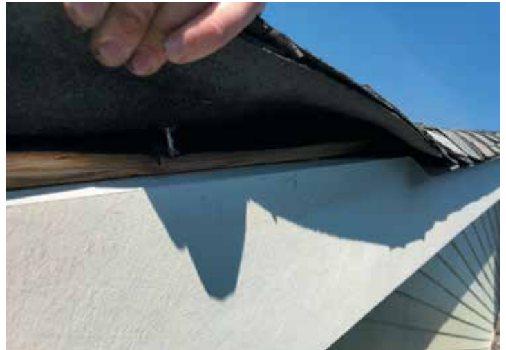
Figure 4. Nailing missed sheathing, no edge metal present per codes, excessive shingle overhang—all of which violate manufacturer's installation instructions.
