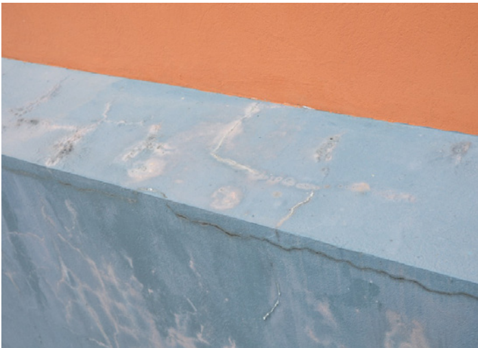
FIGURE 9. Stucco on water table is cracked.
