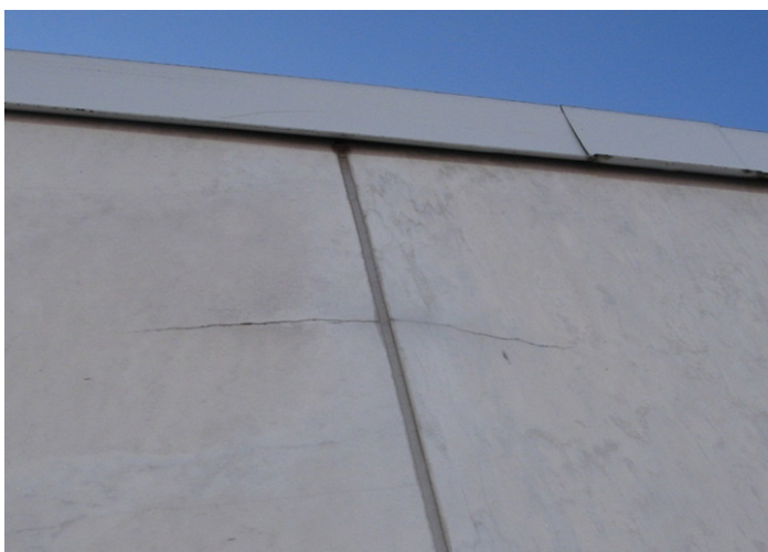
FIGURE 13. View of typical cracking of panels.
