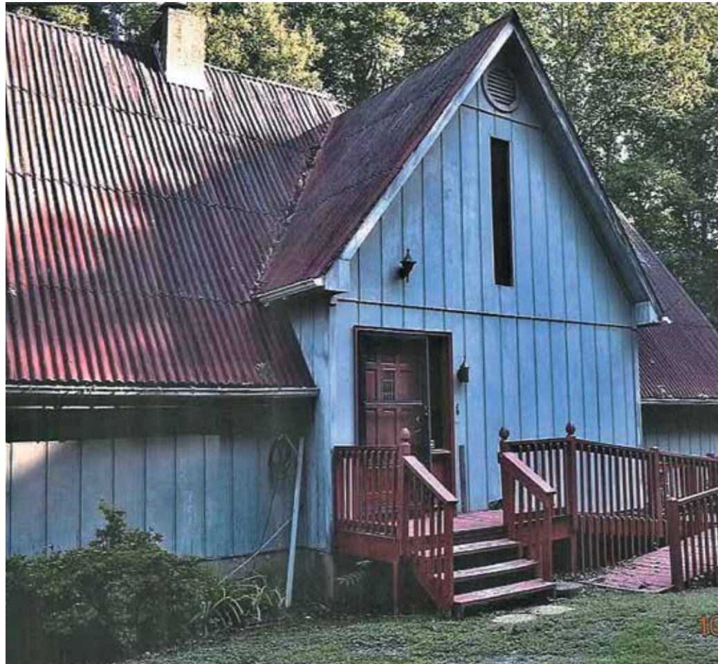
Figure 2. This steeply pitched asbestos-panel roof has served for decades.
