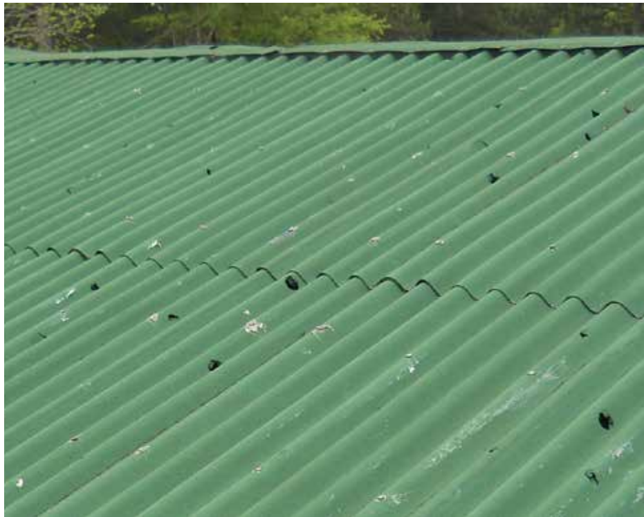
Figure 3. This corrugated fiber-reinforced polymer roof sustained impact damage from hail exposure. Materials should not be applied on top of this roofing product.
