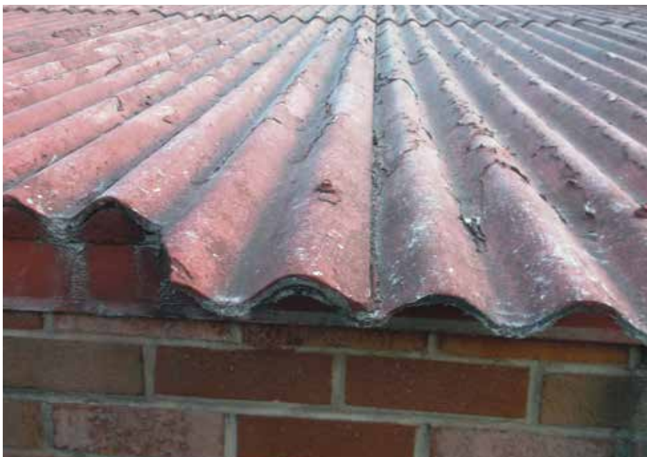
Figure 1. Corrugated asbestos panels are a vintage product that were widely used as siding and roofing materials alike. They are inappropriate for use as the substrate for over-roof assemblies.
