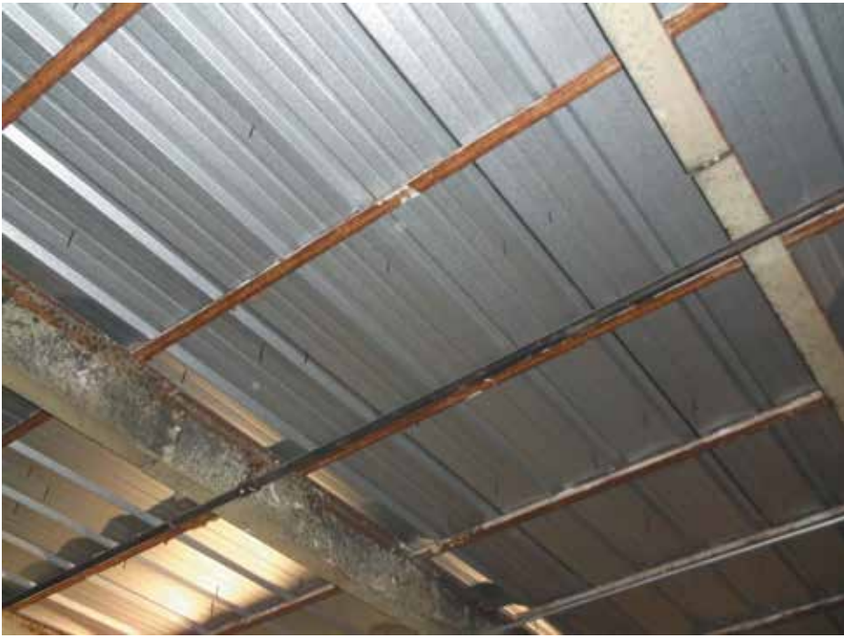
Figure 4. Ordinary ribbed metal panels are situated over iron bulb-tee rails left in place following removal of the old gypsum deck.
