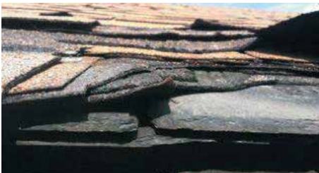
Figure 5. Two layers of asphalt shingles over a slate roof. It is perplexing to consider what the installer was thinking as nails were being driven.
