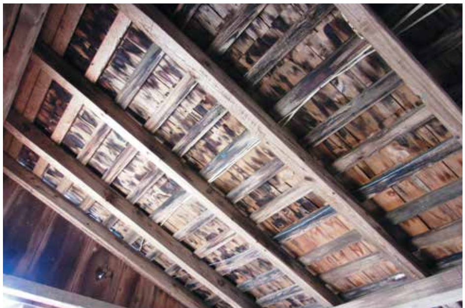
Figure 8. Wood shakes can perform very well over skip sheathing. However, this form of roofing is not a suitable substrate for any additional layers.
