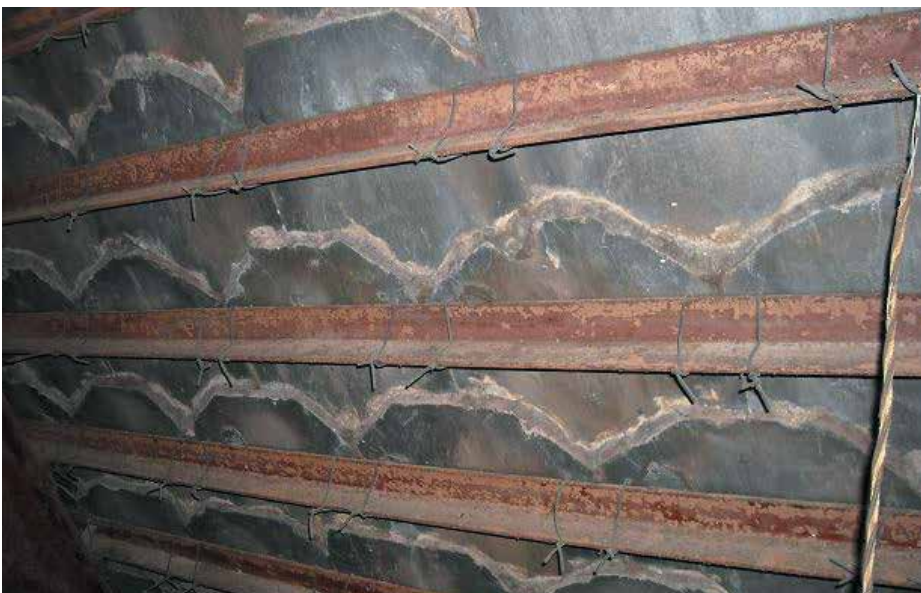
Figure 6. Slate roofs can sometimes be found wired down to iron framing. Slates are not suitable for receiving any kind of additional material.
