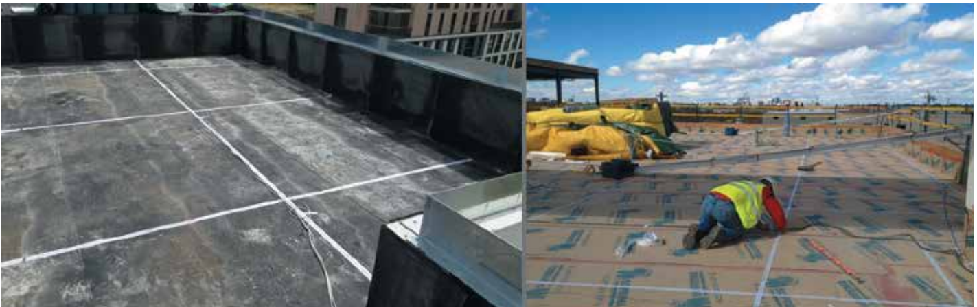
Figure 8. Moisture detection sensors being installed on a vapor barrier and a vapor retarder.
