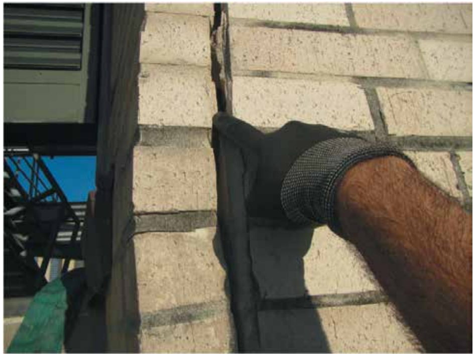
Figure 5. Arm's-length review of noted parapet distress.
