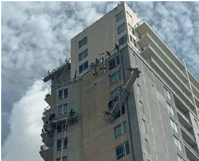
Figure 1. Swing stage collapse in Houston, TX.
