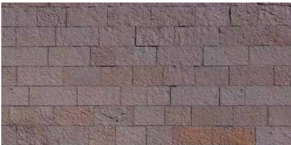
Figure 7. Screenshot of photomesh used to assess stone cladding. Photomesh was used in conjunction with manual assessment, removals, and lab testing. Photomesh was also used to develop drawings labeling each individual stone on the building.
