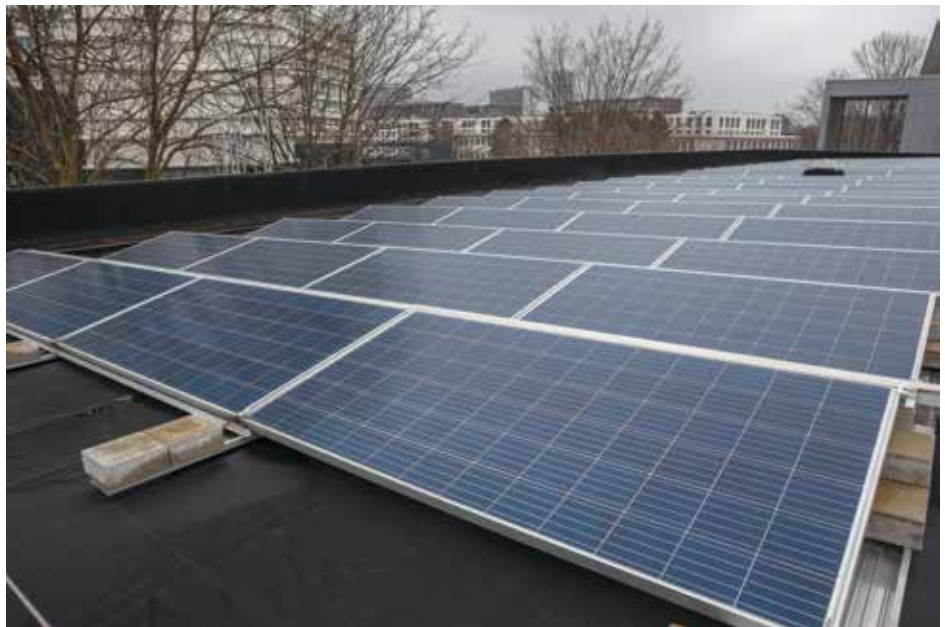
Figure 7. Ballasted solar racking system.
