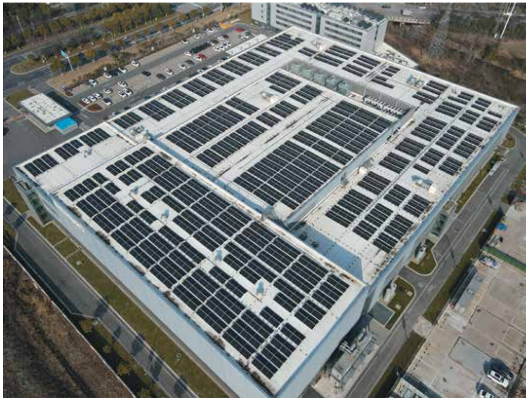
Figure 1. Rooftop solar project.
