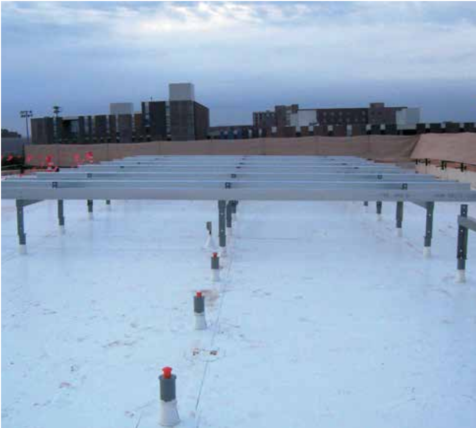
Figure 8. Mechanically attached solar racking system.
