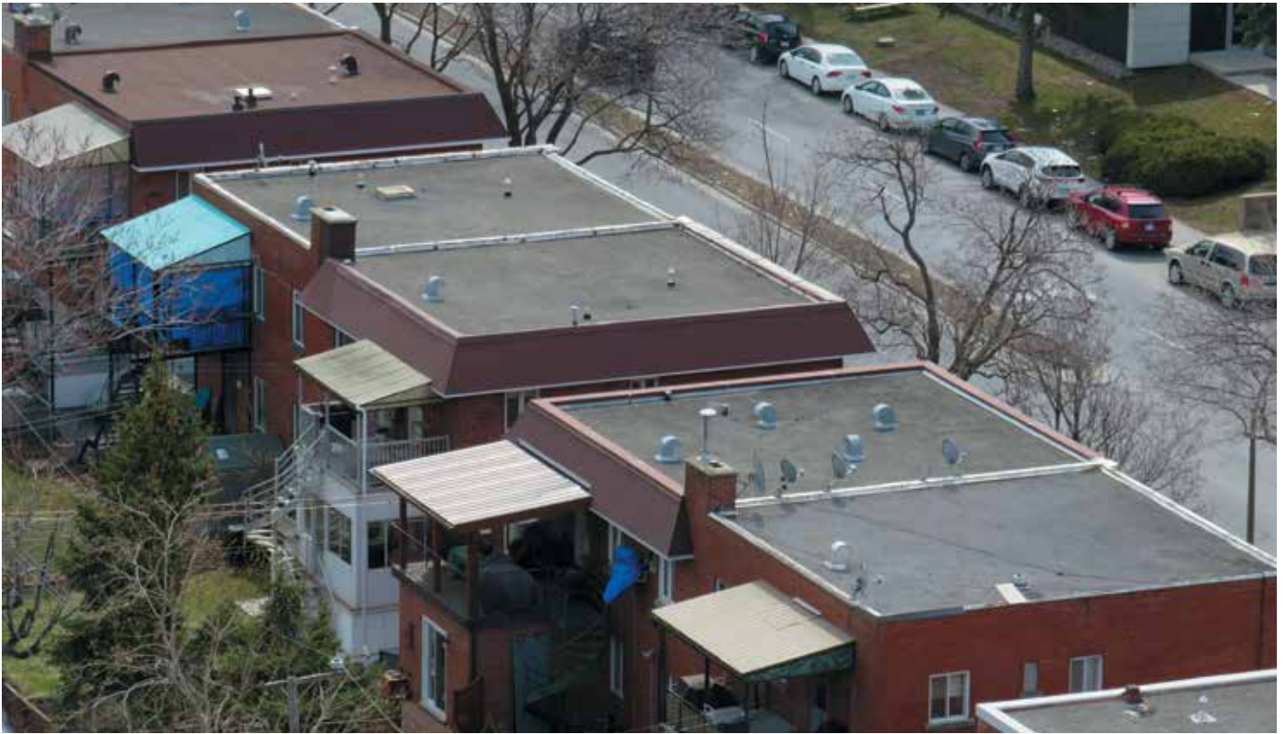
Figure 1. Various roof ventilation strategies employed for similar roofs in the Villeray/Parc-Extension borough of Montreal.
