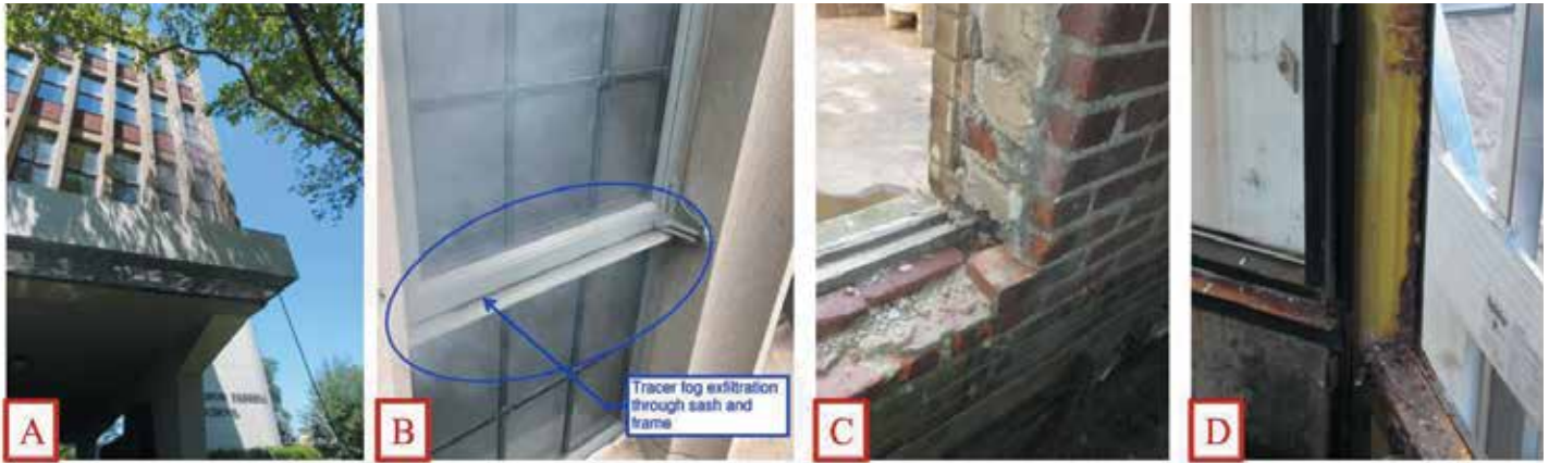
Figure 1. Invasive and noninvasive investigative procedures. (A) Water testing; (B) Tracer fog air infiltration testing; (C) Invasive opening at masonry; (D) Invasive opening at steel framing.
