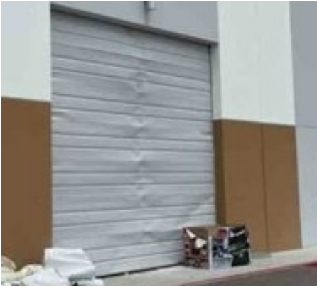
FIGURE 4. Garage door damage, showing distortion from winds at or below 64 mph.
