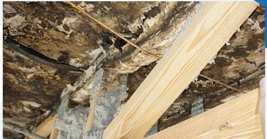
FIGURE 1. Sheathing and truss failure in insulated roof framing system (insulation removed to show distress).
