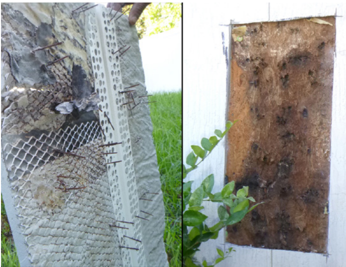
FIGURE 3. Example of damage resulting, at least in part, from the fastening down of the control joint accessory.
