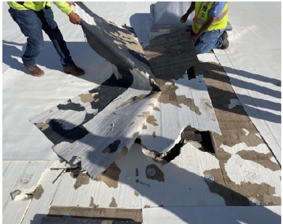
FIGURE 5. Fractured ISO with fasteners and membrane intact.
