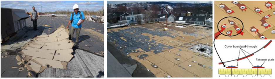
FIGURE 15. Substrate pullout from the fastener and plate for a PARS.
