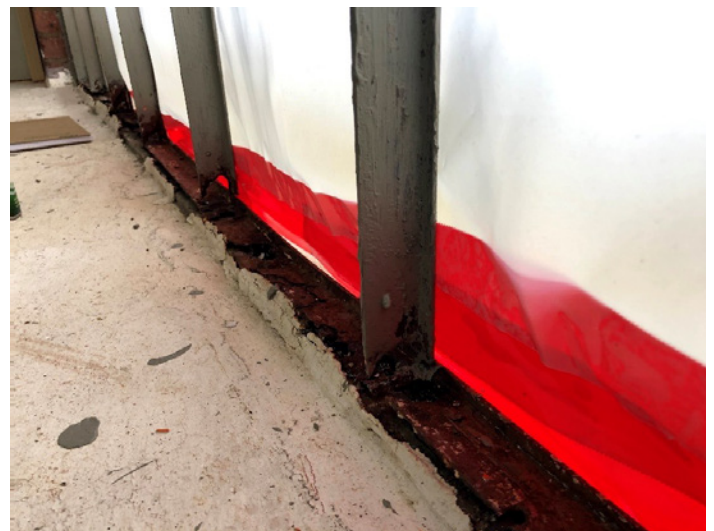
FIGURE 2B. Coating removal reveals extensive corrosion of steel mullions.
