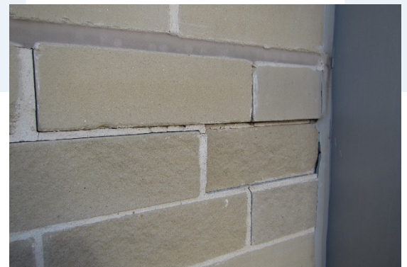
FIGURE 3. Extensive mortar cracking as observed in the Phase 3 investigations.
