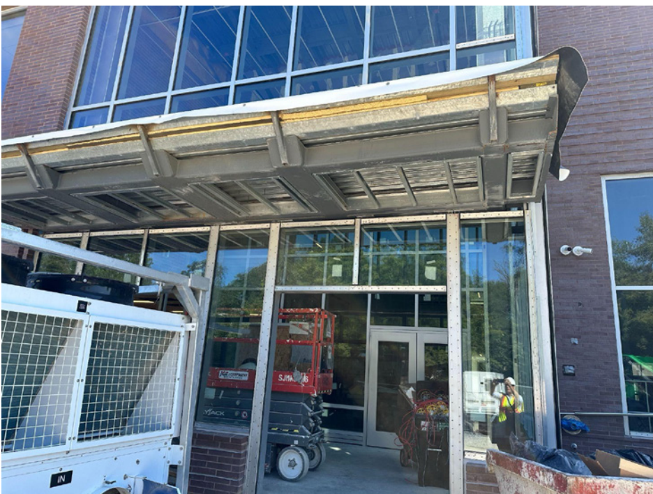
FIGURE 3. Canopy transition condition that is frequently a source of air leaks during a whole building airtightness test.
