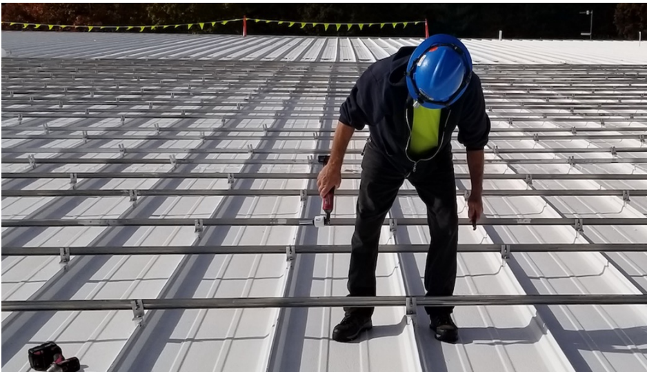
FIGURE 1. Flush Rail Mounting; Use of rails on the metal roof is redundant, and adds unnecessary collateral load.
