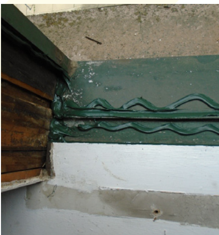
FIGURE 6. One-off fenestration replacement where the perimeter air/water barrier is limited to sealant.
