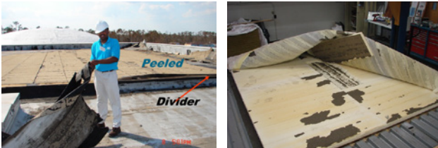
FIGURE 16. Facer delamination failures for an AARS.
