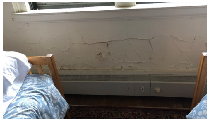
FIGURE 5. Interior finish damage beneath fenestration was caused by water accumulating between the storm window and the original fenestration unit.
