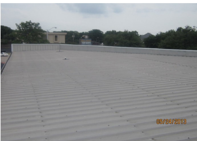
FIGURE 9. Photograph of the case study roof taken in 2013, approximately 18 years after the hail event, when the roof was 27 years old.
