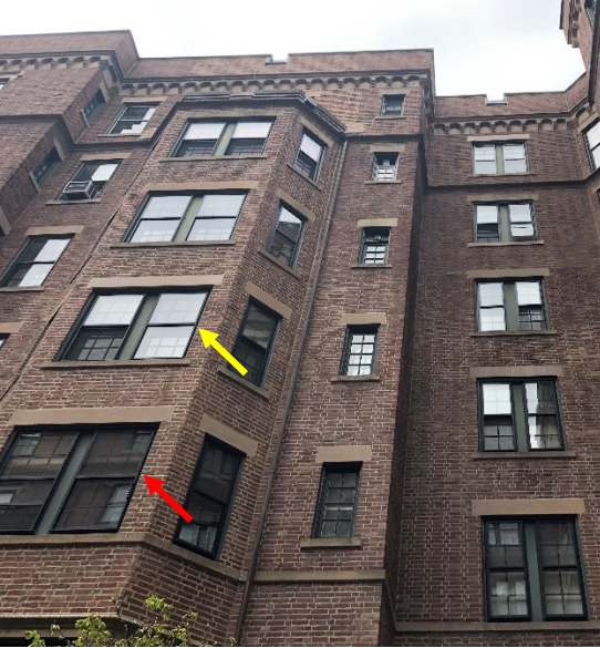
FIGURE 1. Figure 1. Storm windows installed at localized fenestration of a condominium building. Yellow arrow indicates a location with a storm window, red arrow indicates a location without a storm window.
