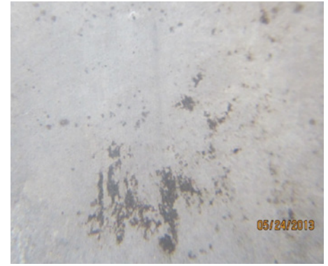
FIGURE 13. Photograph of a cleaned hail-caused dent under 10x magnification—note the absence of evident corrosion.
