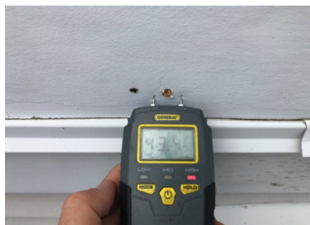
High moisture content within the siding trim.
