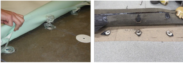
FIGURE 11. Membrane pullout from the fastener plate in MARS.
