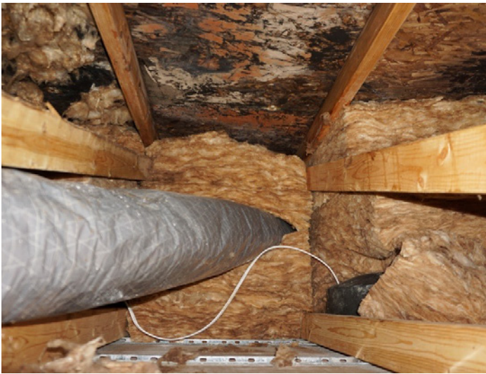
FIGURE 3. Ductwork within insulation.
