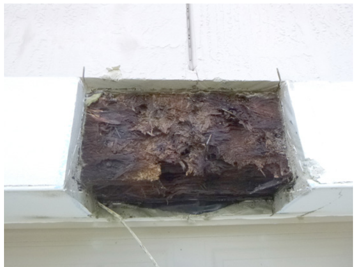
FIGURE 6. Example of damage resulting, at least in part, from a missing weep accessory at the horizontal-to-vertical intersection.
