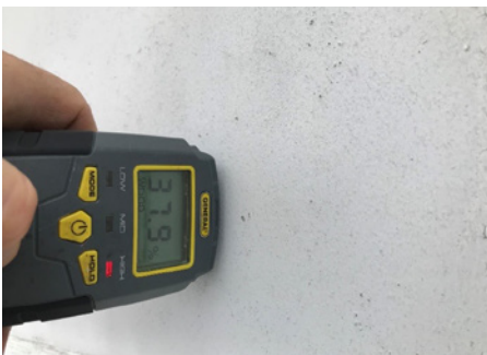
High moisture content within the siding trim.
