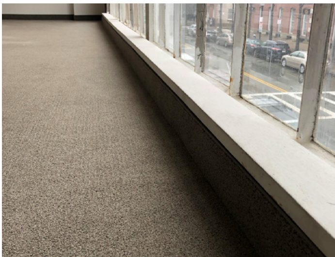
FIGURE 2A. Coating and glazing putty conceal corrosion of steel mullions.
