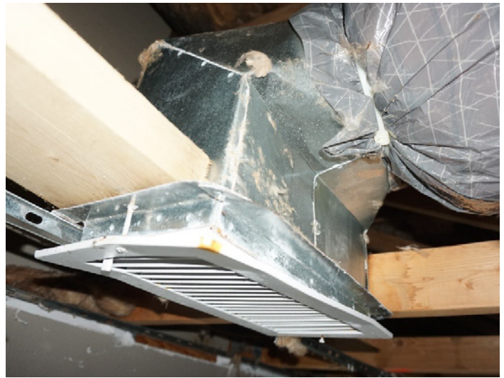
FIGURE 4. Zip tie connection of flexible duct to ceiling diffuser.
