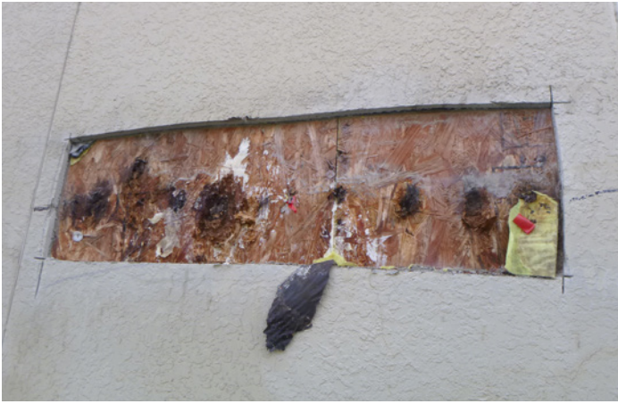
FIGURE 1. Example of damage resulting, at least in part, from fasteners installed between framing members.
