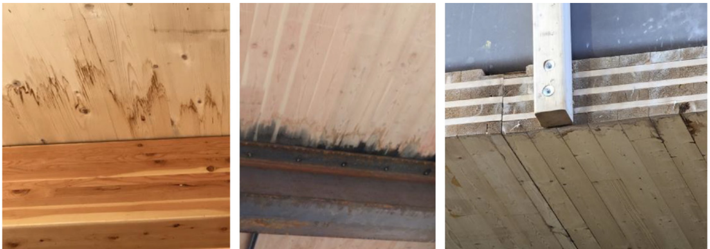
FIGURE 8. Damage due to moisture exposure from the 2023 RDH Building Science Laboratories evaluation. 11
