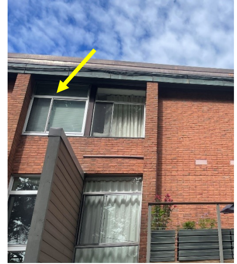
FIGURE 3. Sightlines at the replacement fenestration (indicated with the arrow) are thicker than existing fenestration profile next to it.
