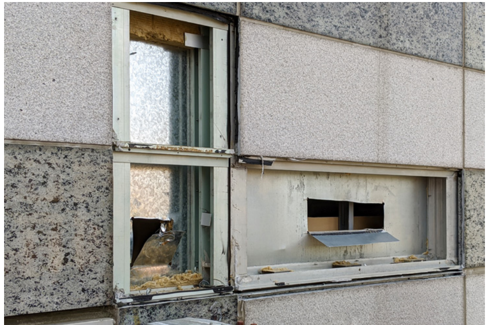
FIGURE 7. Existing Unitized Curtain Wall and Glazed in Granite Panels – Credit Jensen Ying.
