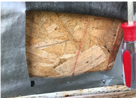
Mildew found on the surface of the OSB sheathing behind the building wrap.
