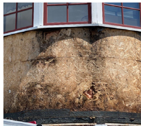
A large percentage of sheathing was rotten and had mold growth from high moisture content stemming from the wall assembly. Additionally, insulation within multiple bays and some wall studs was wet and saturated. This wall assembly is the same as the rest of the school.
