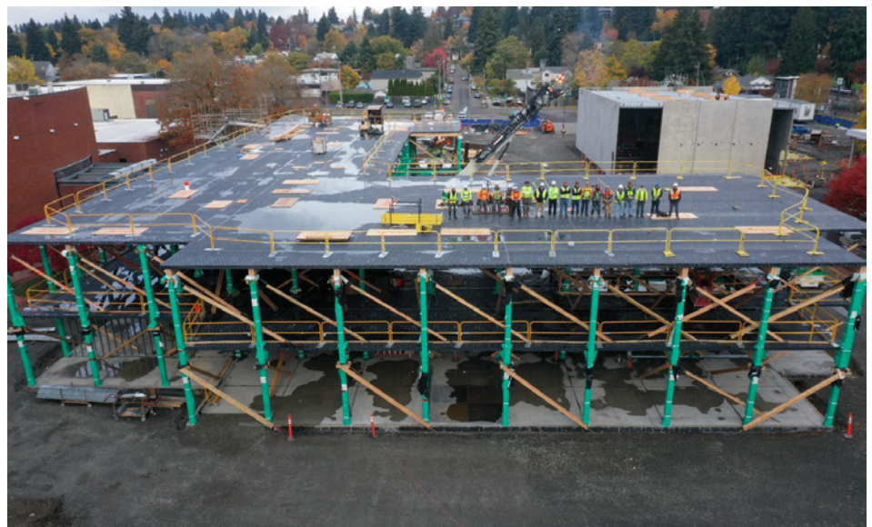
FIGURE 10. Moisture protection applied to the CLT floors as a vapor permeable self-adhered membrane and glulam columns using a vapor permeable membrane wrap.
