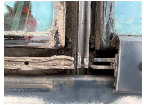
FIGURE 3. Skylight with overlapped raised drainage channels.
