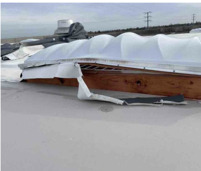
FIGURE 2. Curb and skylight separation from the deck.
