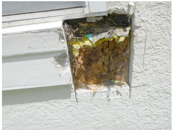
FIGURE 4. Example of damage resulting, at least in part, from improper separation between window and stucco.
