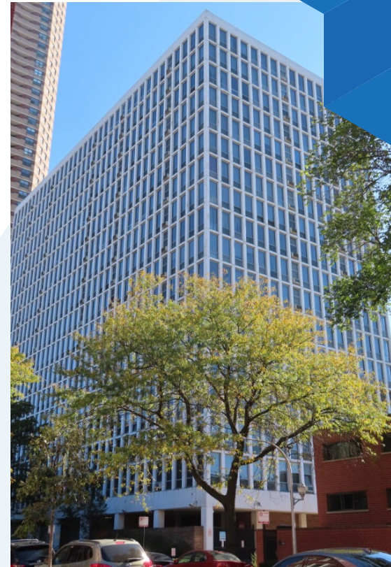
FIGURE 1. Building Exterior Walls Consisting of Concrete Columns, Concrete Slab Edges, Windows, and Sealant Joints.
