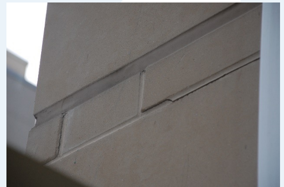
FIGURE 2. Loose stone observed as part of the initial investigation reports.
