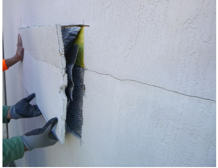
FIGURE 2. Example of damage resulting, at least in part, from lath not installed backing on backing and metal on metal.
