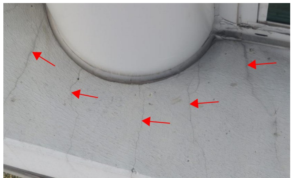
FIGURE 8. Cracks at Concrete Skyward-Facing Surface Extend Below Sealant Joints.
