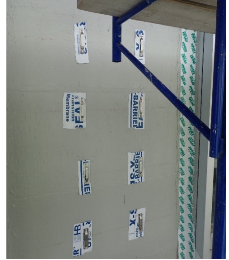
FIGURE 7. Installation of new sheathing, air barrier, and brick ties during masonry re-clad.
