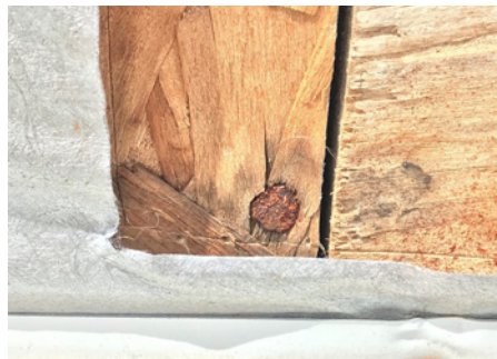
Rusting nail head behind the building wrap.
