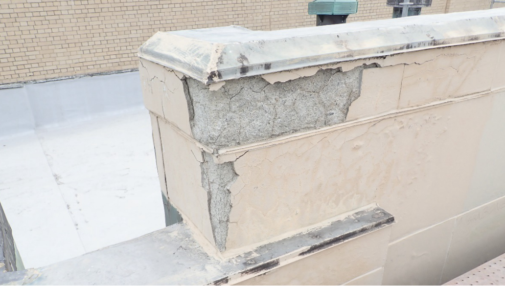
FIGURE 3. Cast stone units at the parapet with freeze-thaw damage and coating failure. Source: Wiss, Janney, Elstner Associates Inc.
