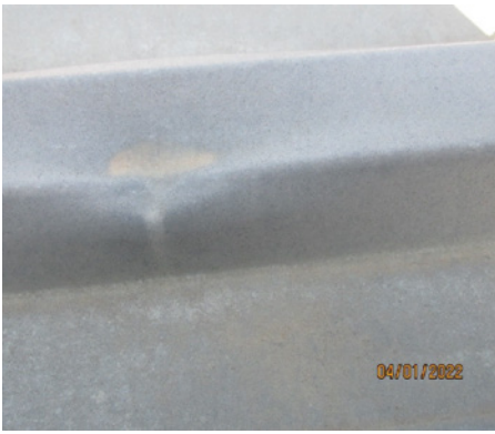
FIGURE 15. Photograph of large dent in the rib of the panel.
