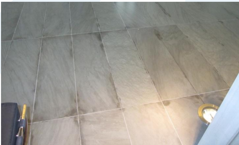
FIGURE 1. Permanently stained interior flooring from moisture exposure.
