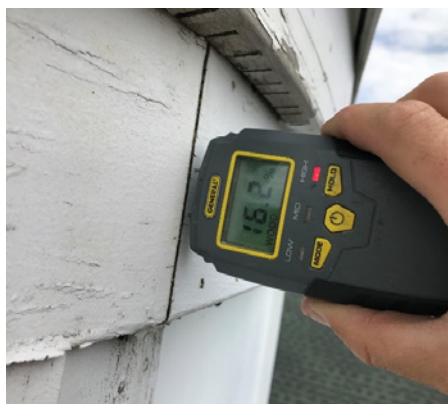
This high moisture reading was taken in an area that was replaced in 2021. The reading was taken in 2019 at the trim and the photo to the right shows the condition of the sheathing behind the air barrier that was uncovered prior to a new rainscreen wall assembly system being installed.
