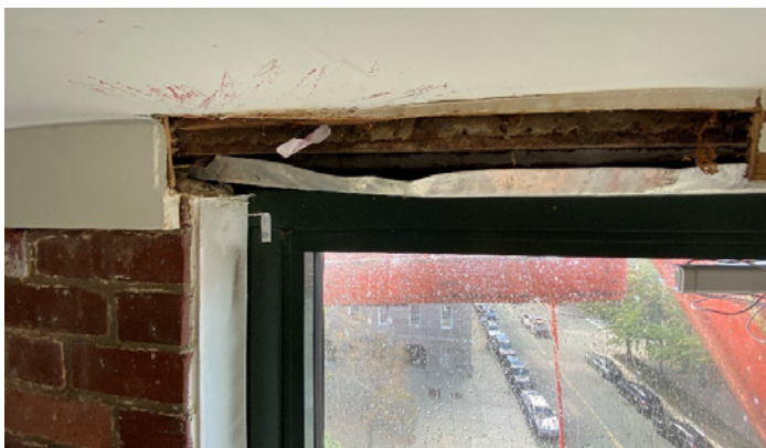
FIGURE 4. Water leakage at interior appears at window head; however, the leakage path is through exterior masonry wall above.
