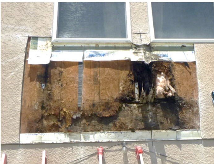
FIGURE 5. Example of damage resulting, at least in part, from improper separation between window and stucco.
