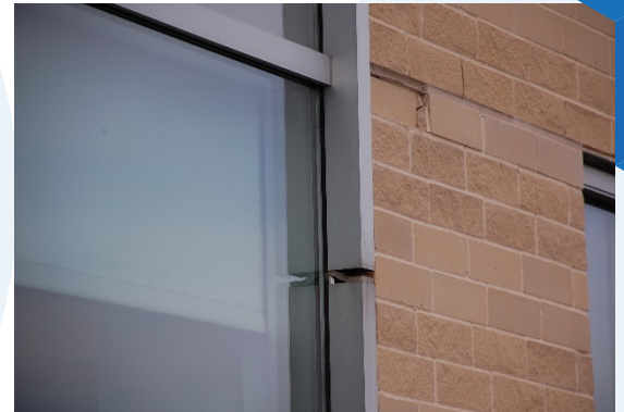
FIGURE 1. Dislodged stone observed as part of the initial investigation reports.
