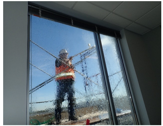
FIGURE 9. AAMA 501.2 nozzle water testing was performed at a punch window in order to evaluate potential water leakage
