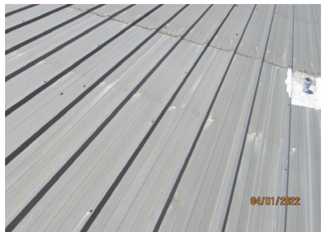
FIGURE 14. Photograph of case study roof taken in 2022 approximately 17 years after the Mayfest Storm.
