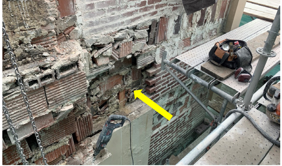
FIGURE 6. The removal of cast stone units from the sanctuary facade exposed structural clay tile back-up masonry. Note the void where 8-in.-deep (203-mm-deep) units were removed (arrow). Source: T. Ikenouye, Wiss, Janney, Elstner Associates Inc.
