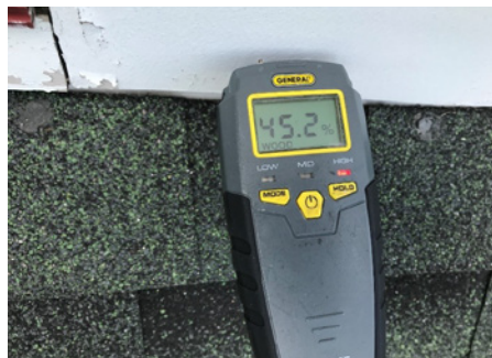
High moisture content within the siding trim.
