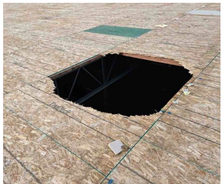
FIGURE 3. Loss of rooftop curb due to possible internal pressurization.
