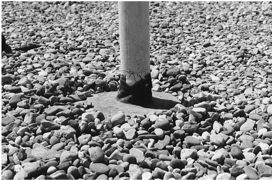
Photo 12: Stress on accessory due to membrane shrinkage.
