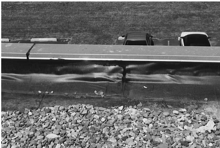
Photo 13: Stress on termination due to membrane shrinkage.
