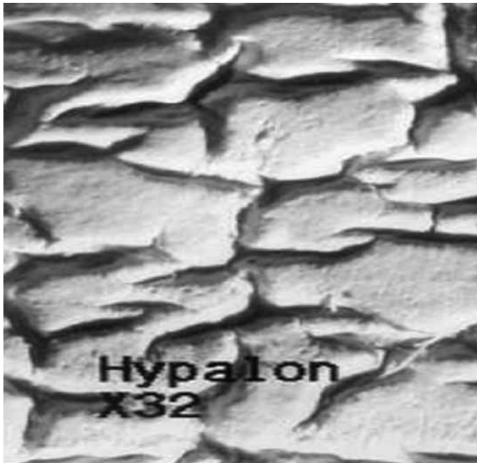
Figure 10: Surface deterioration of a thermoplastic single ply.
