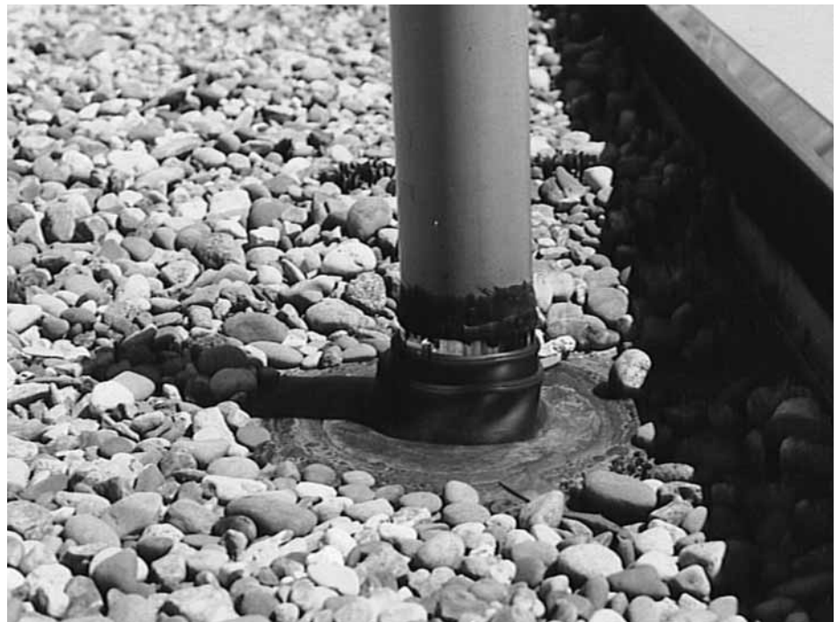
Photo 11: Stress on accessory due to membrane shrinkage.
