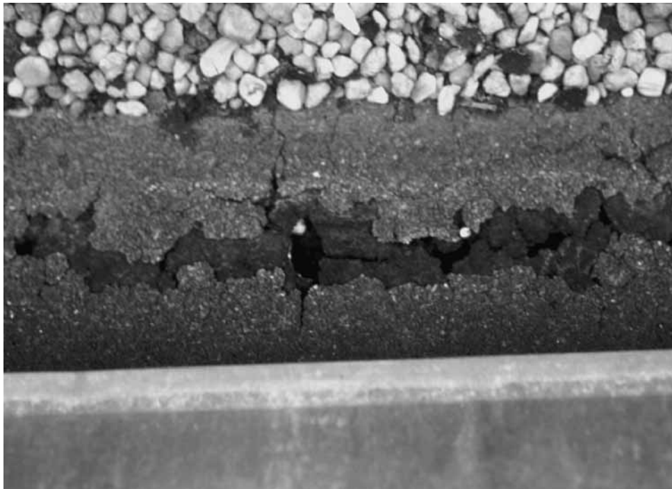
Photo 8: Degraded base flashing.
