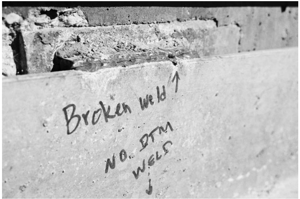
Figure 23 – Broken weld at shelf angle attachment.
