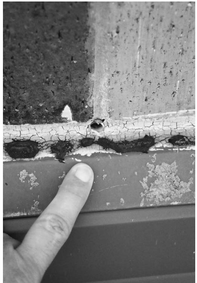
Figure 18 – Flashings oozing; weep tube clogged.
