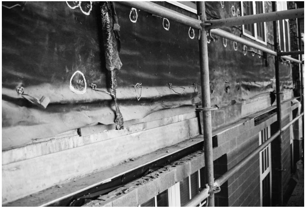
Figure 8 – Weather-resistant barrier not integrated with shelf angle; missing wall ties.
