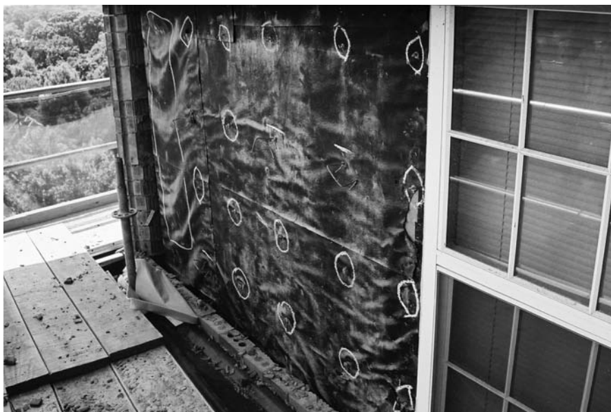
Figure 13 – Missing wall ties at one section of wall.
