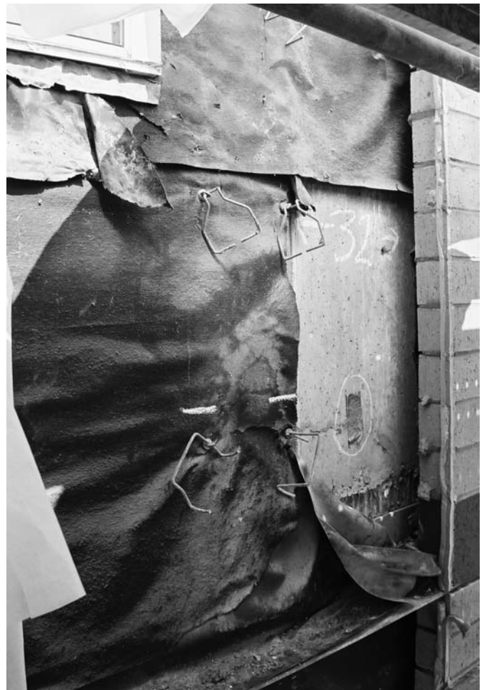
Figure 9 – Weather-resistant barrier stops short of column; not sealed at terminations.
