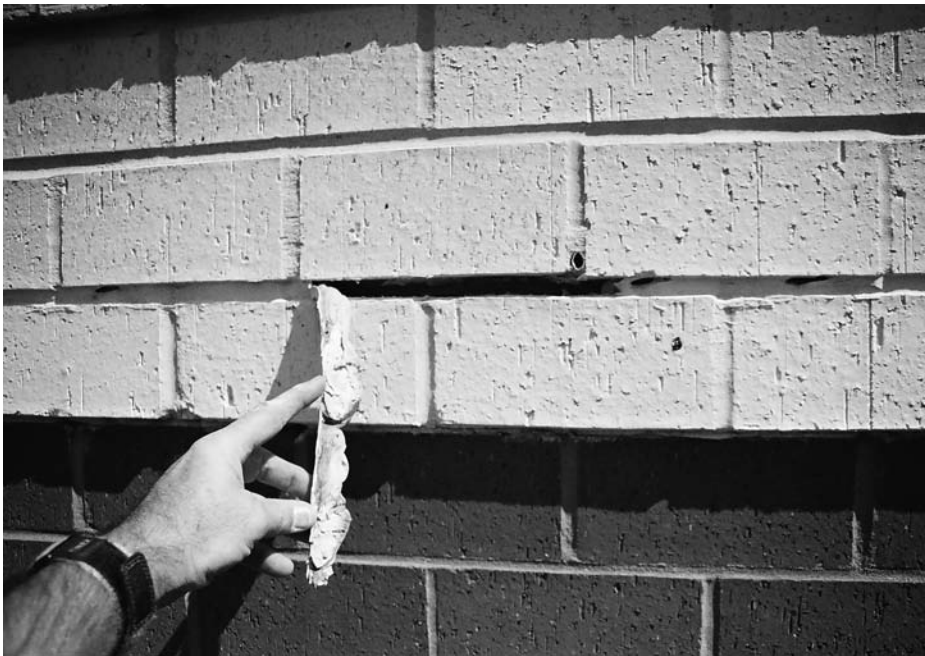
Figure 5 – Sealant installed with no backer rod.
