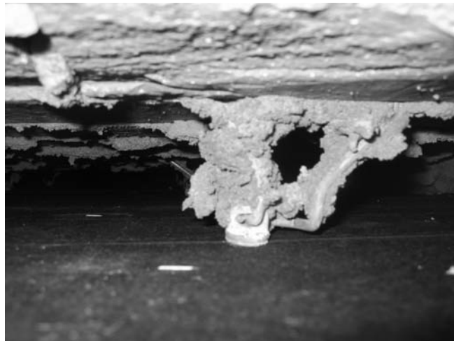
Figure 20 – Mortar bridging at wall tie.
