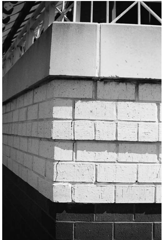
Figure 2 – Cracks in brick veneer at corner.
