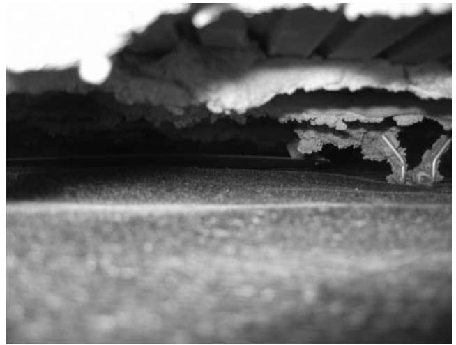
Figure 19 – Mortar bridging at wall tie.
