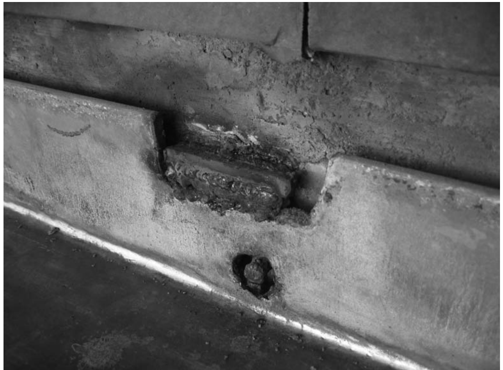
Figure 22 – Improper weld between shelf angle and embed.
