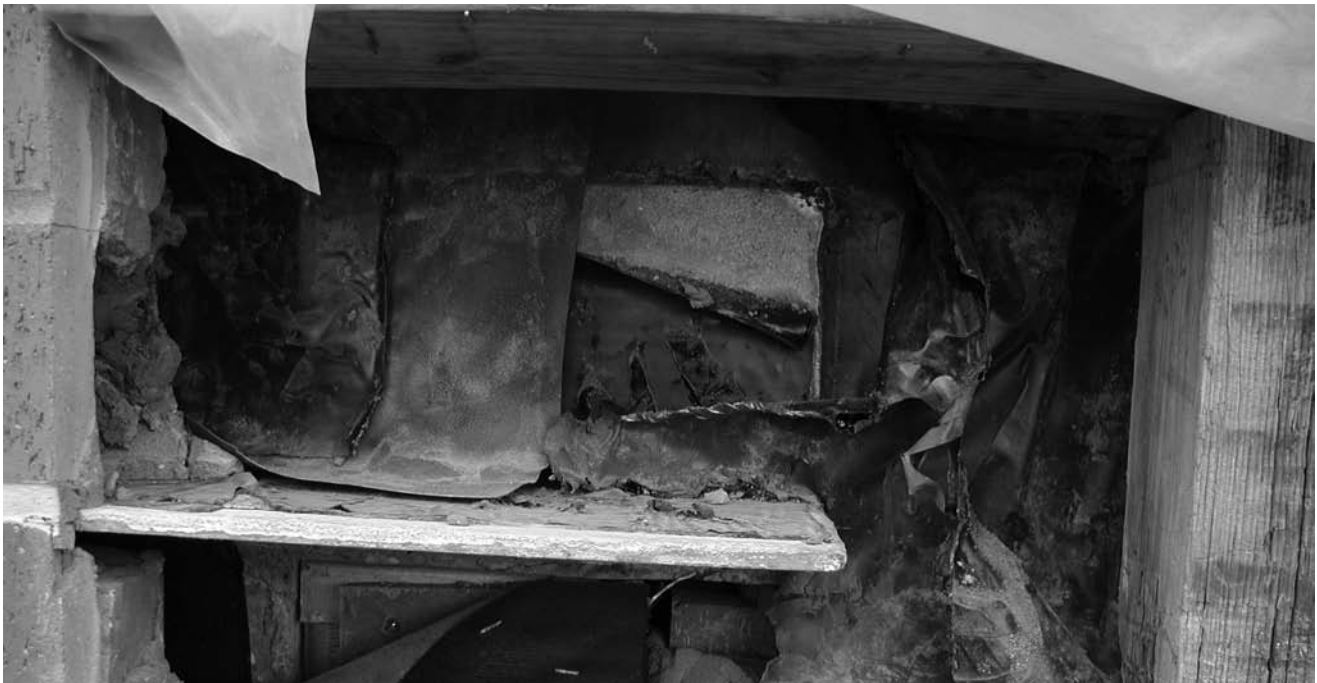
Figure 15 – Shelf angle offset in elevation; no end dam at membrane flashing.
