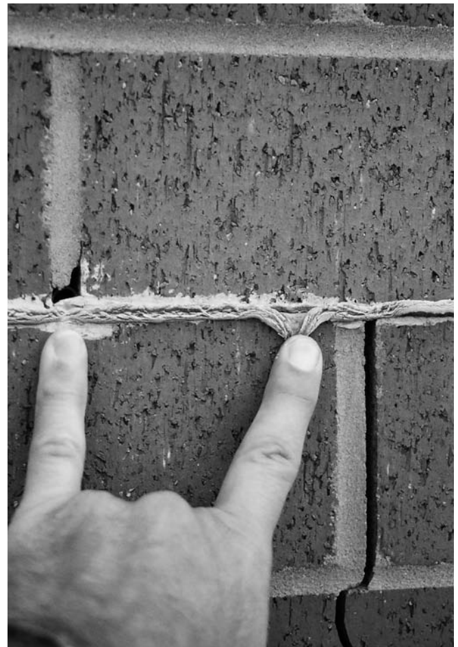
Figure 6 – Sealants failing in compression: masonry cracks.
