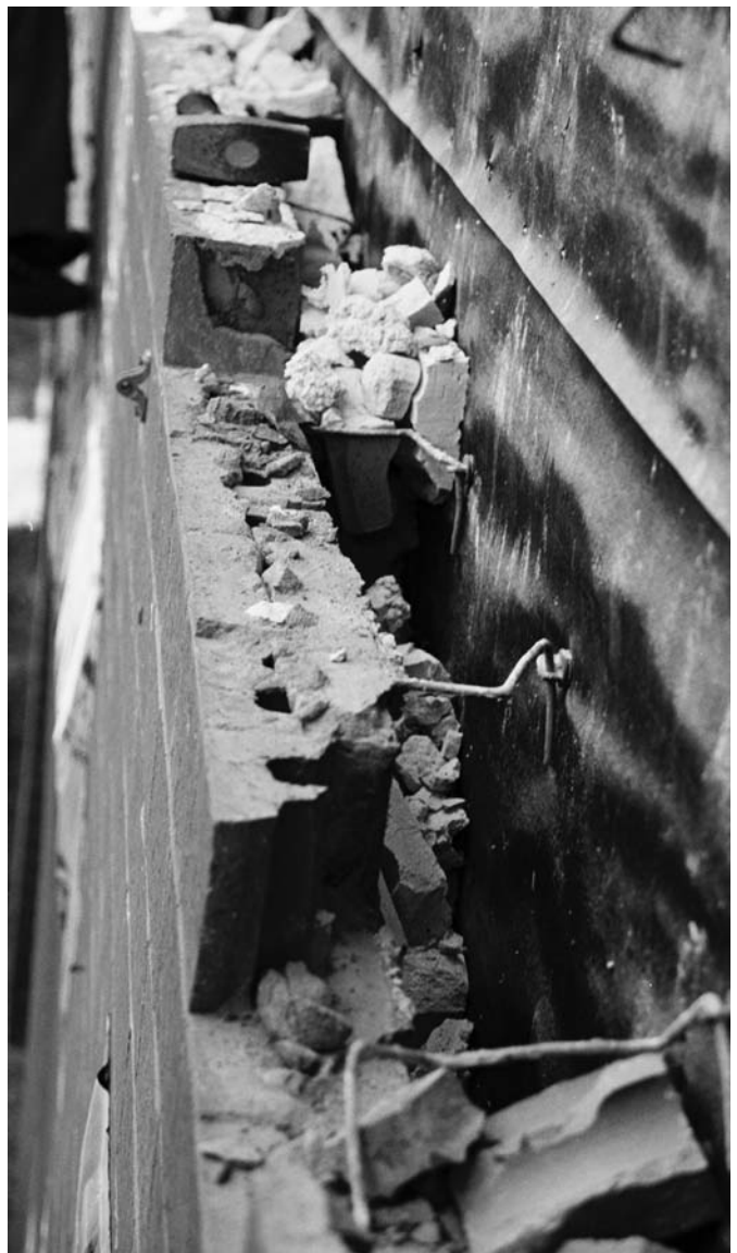
Figure 12 (above) – Wall ties improperly installed with one leg engaged.
