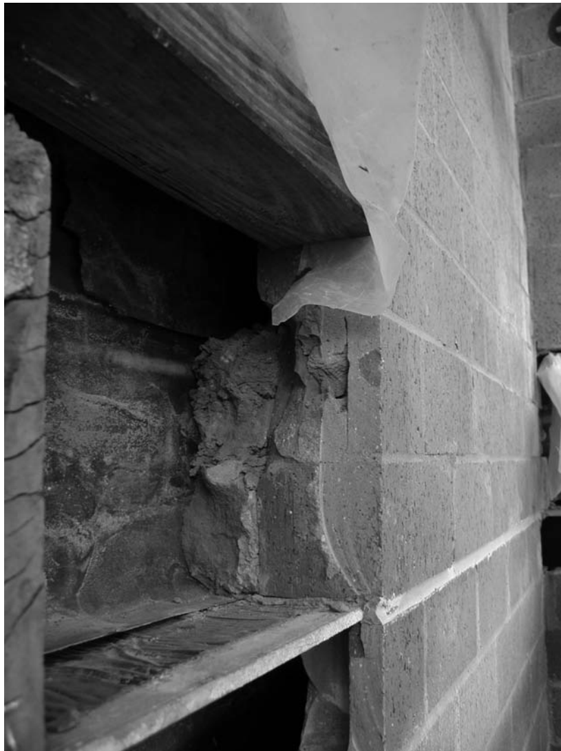
Figure 21 – Excessive mortar droppings in drainage cavity.
