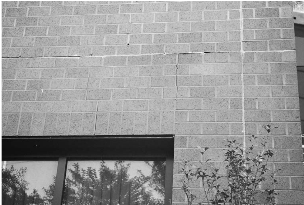
Figure 3 – Cracks in brick veneer above window.
