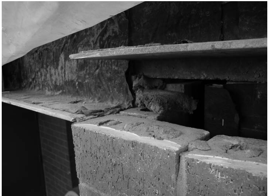
Figure 14 – Shelf angle offset in elevation; no end dam at membrane flashing.
