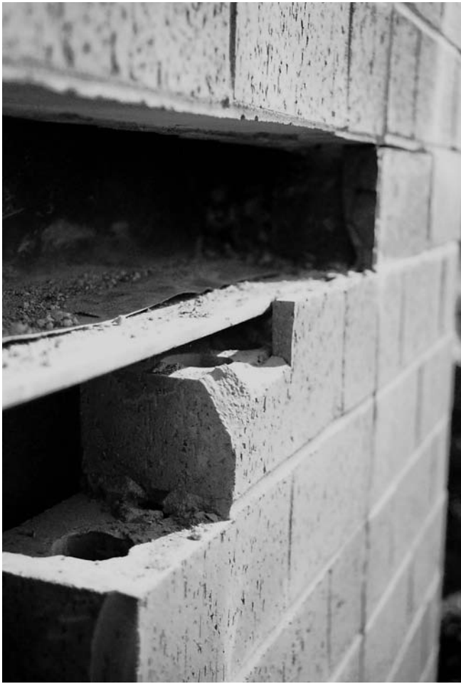
Figure 17 – Coordination error in shelf angle placement; back of brick saw-cut.
