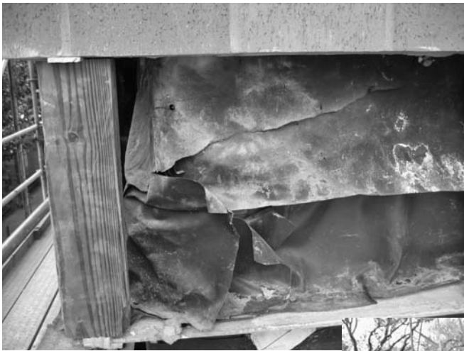
Figure 10 – Improper weather-resistant barrier at corner.
