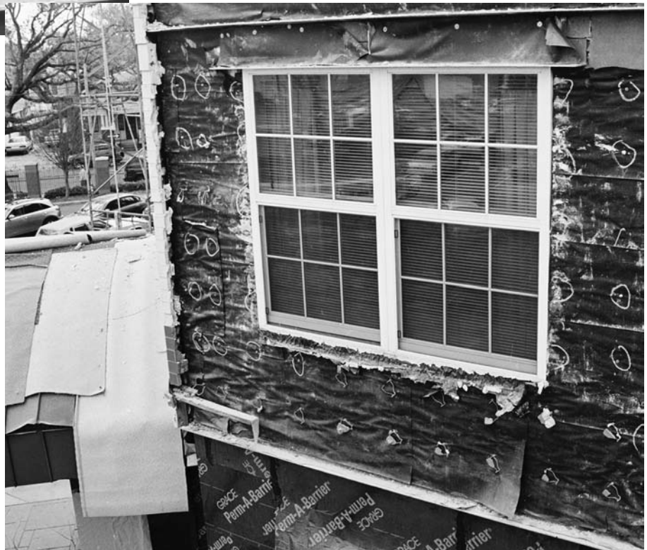
Figure 11 – Missing wall ties at one section of wall.
