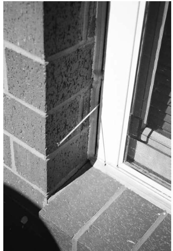
Figure 7 – Adhesive sealant failure at window jamb.
