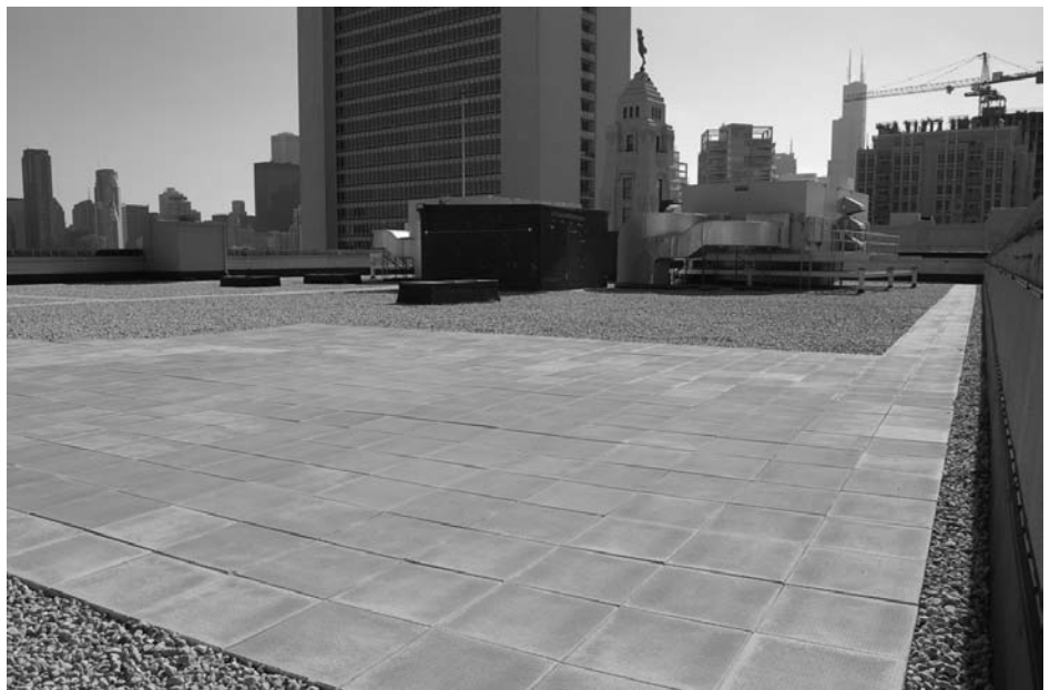
Photo 1 – Recent research by ORNL has found that ballasted systems, both paver and aggregate, provide the same level of energy conservation as do so-called “cool” roof systems.
