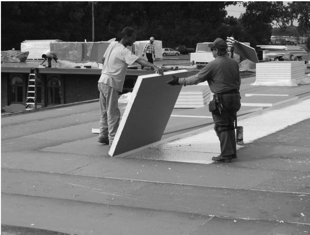
Photo 2 – The use of high levels of thermal insulation is a sustainable methodology in the conservation of energy.
